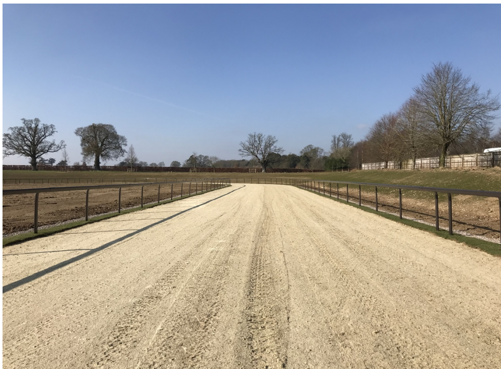
Example of Exercise Track with Duralock fencing.
