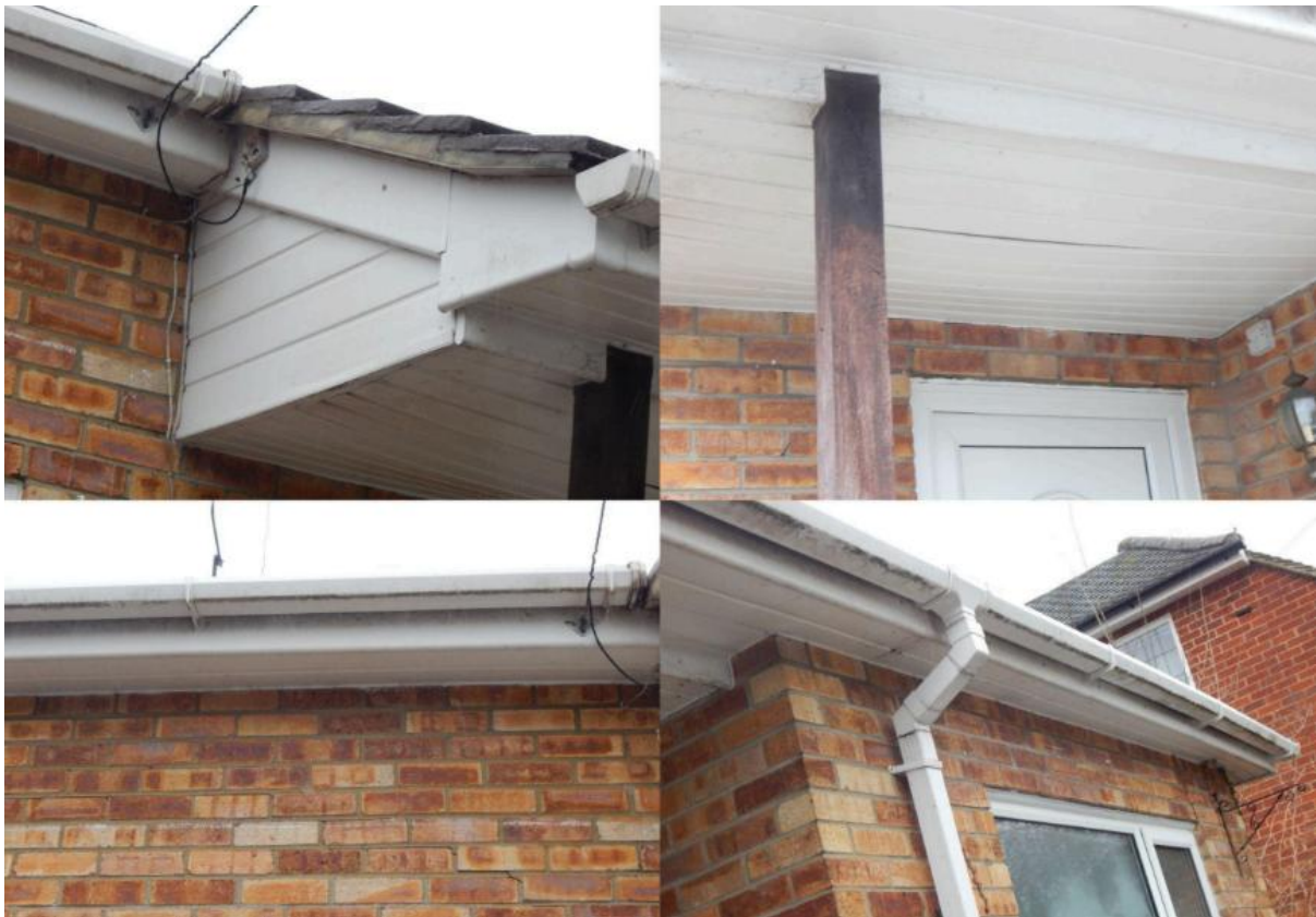
Image 5 – Close views of the eaves coverings to demonstrate condition
