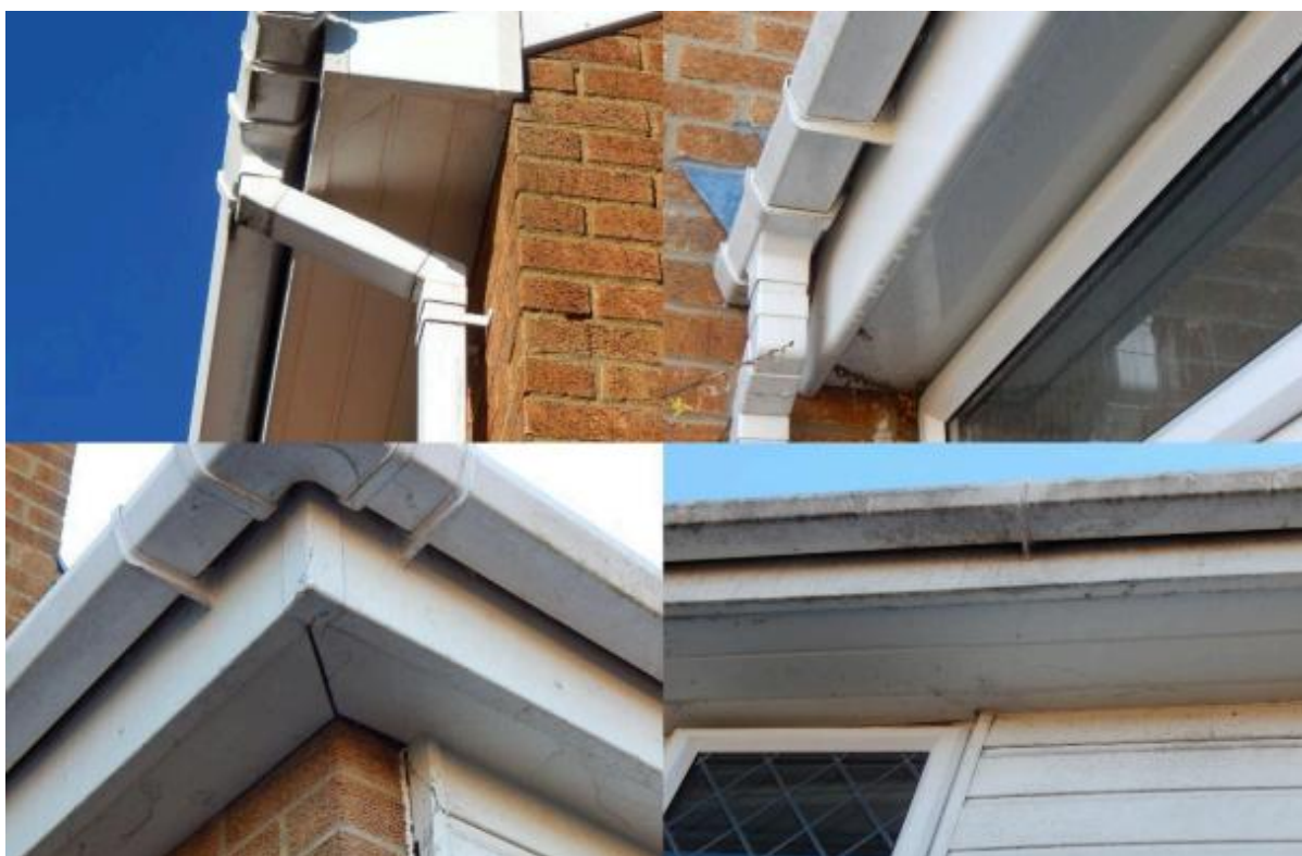
Image 8 – Close view of the eaves coverings to demonstrate condition throughout
