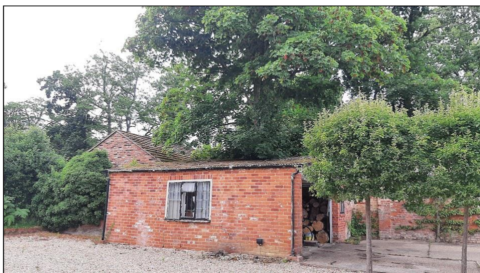
Photograph 17. The southern and eastern aspects of the double garage. Note the large cracks in the brickwork.
