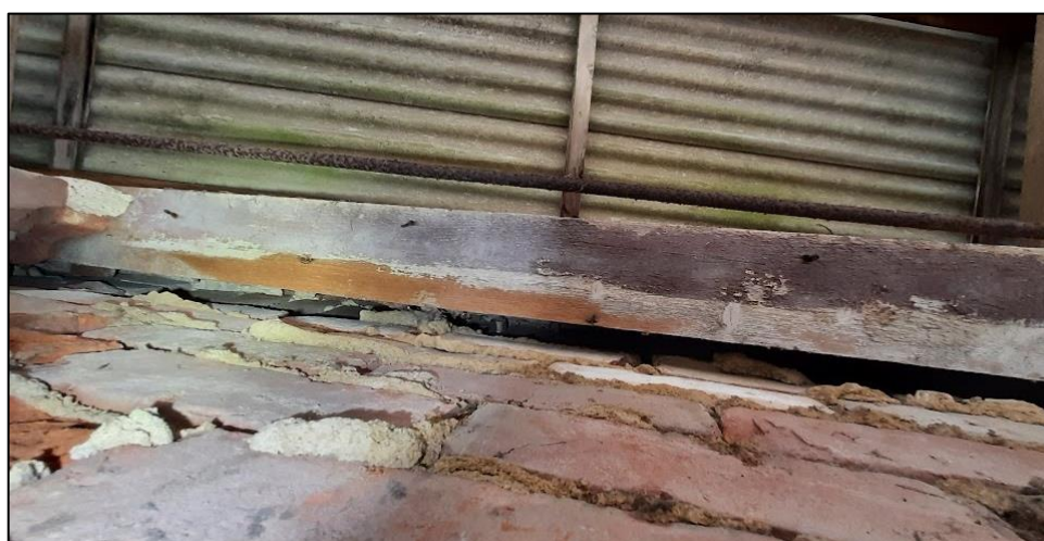
Photograph 12. The horizontal gap to the cavity taken. Picture taken from beneath.
