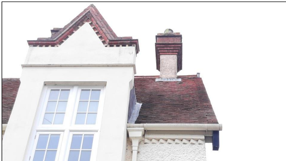
Photograph 4. An example of the gaps identified across the roof of the main house providing suitable bat access and roosting opportunities.
