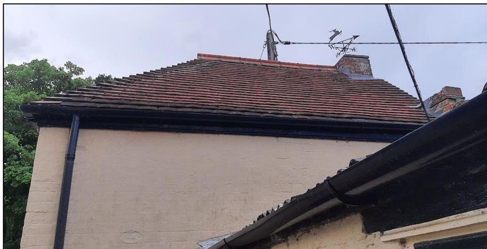
Photograph 15. An example of the gaps identified across the roof of the store providing suitable bat access and roosting opportunities.
