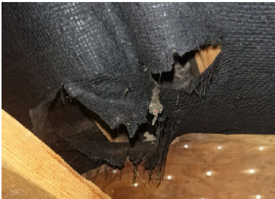
Photograph 11. Tear in bitumen felt with tiles visible behind
