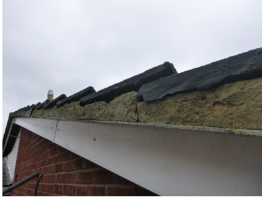
Photograph 5. Crumbling mortar along the verge (southwestern elevation)
