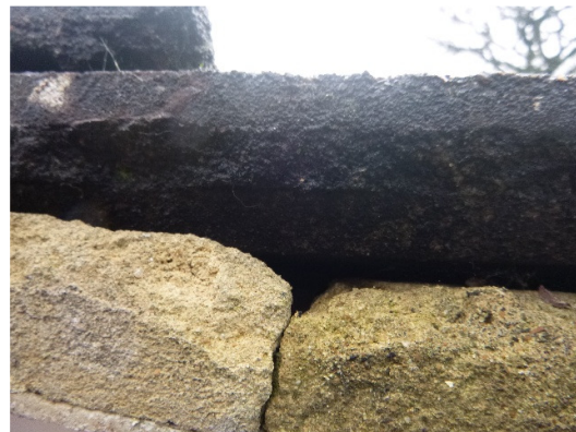
Photograph 4. Verge mortar crumbling; when investigated with endoscope showed no evidence of use by bats (southwestern elevation).
