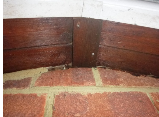
Photograph 6. Crumbling mortar at the apex of the gable end extension which was of limited extent (southwestern elevation)
