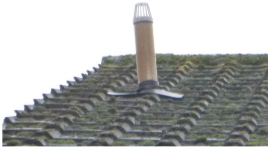
Photograph 7. Gap under lead flashing from flume pipe (front northwest elevation)
