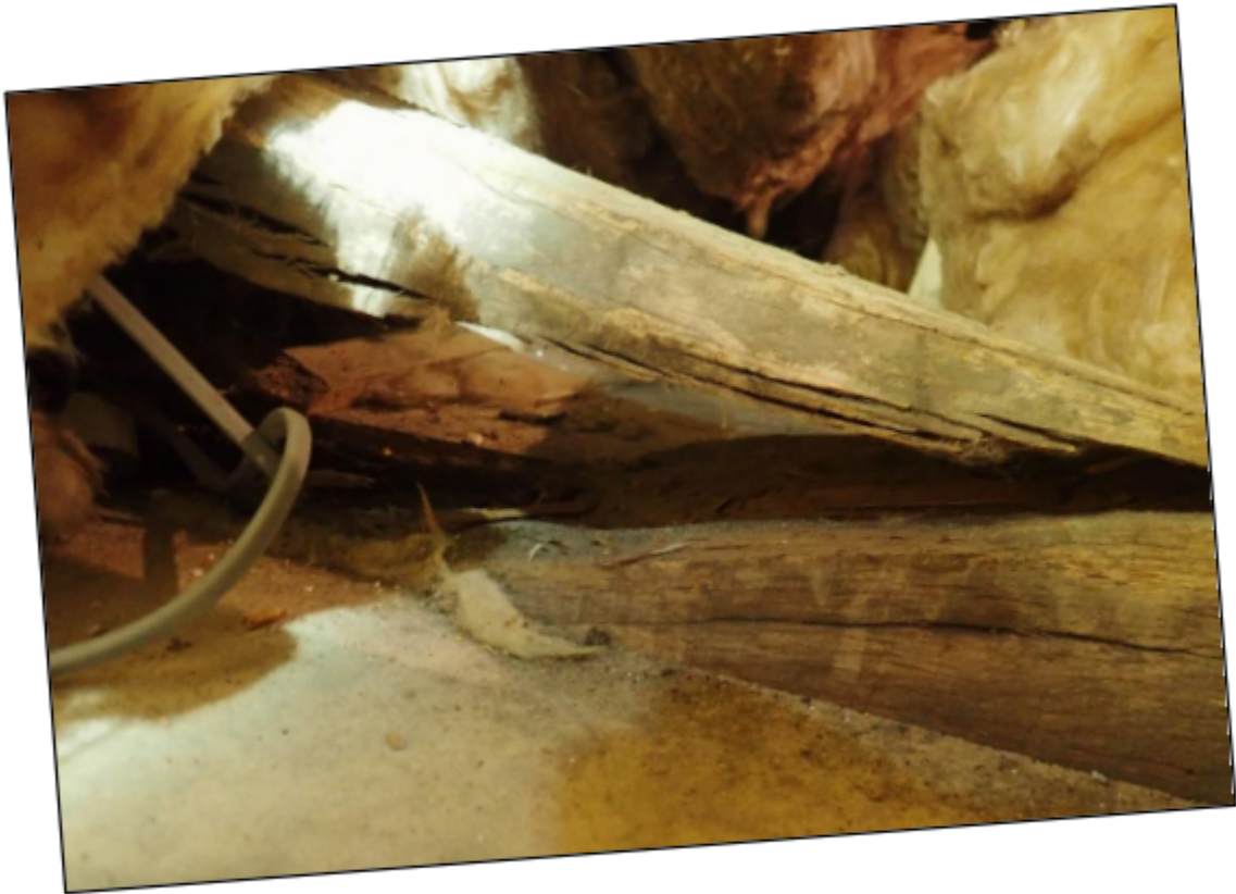
Figure 43. View of the fracture in the 1 st -floor ceiling beam
