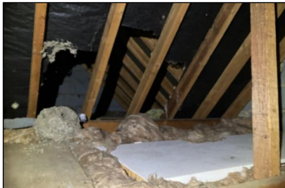
Photograph 6. Old wasps' nest and connectivity throughout the loft void.
