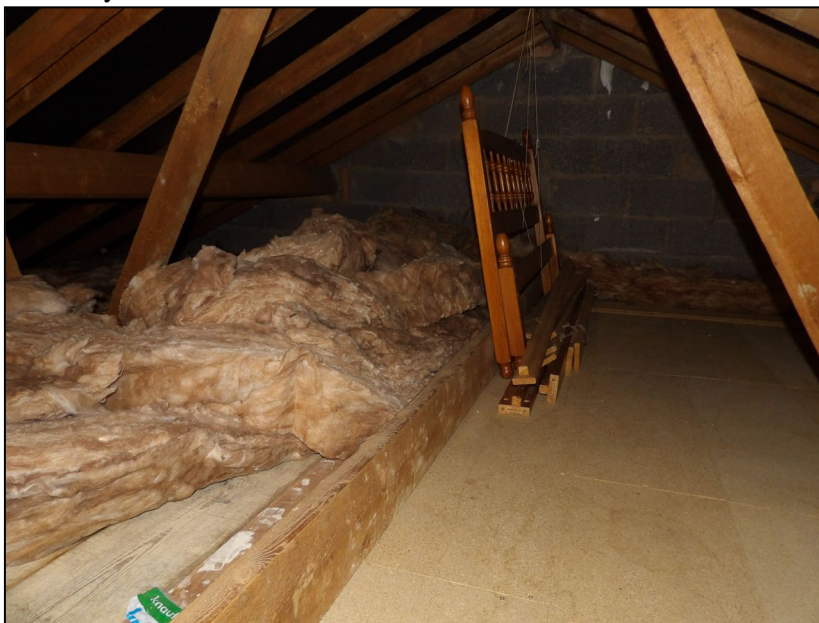
Figure 9. Example of loft space and bitumen felt in property. 11 Retford Close, Woodley. 09.09.25
