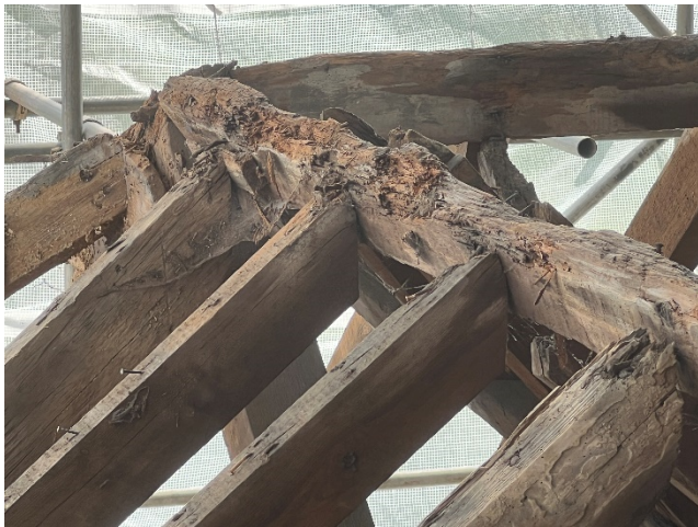
Truss over bedroom 2. (decay at apex)
