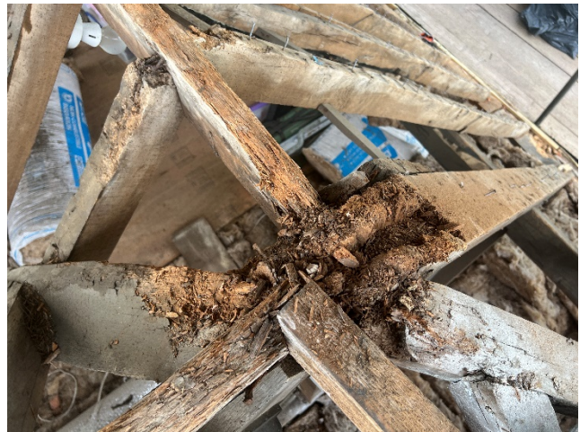
Truss over bedroom 3. (decay to end of king post).
