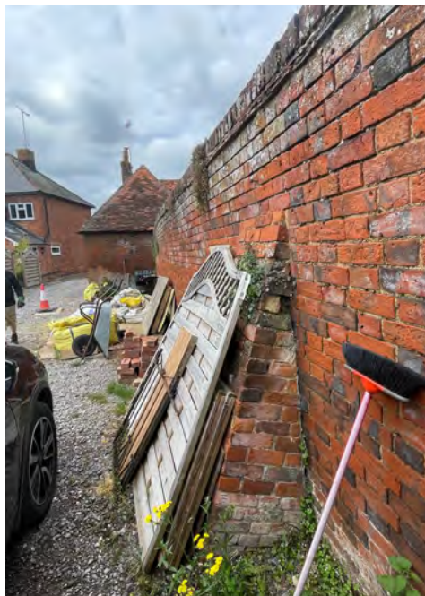
Fig 3.3 Garden wall leaning past the middle third
