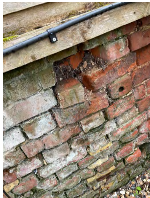
Fig 3.4 Garden wall brickwork in poor condition
