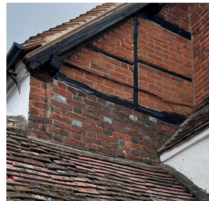
Fig 3.6 Brickwork gable with small crack and brickwork with cement mortar
