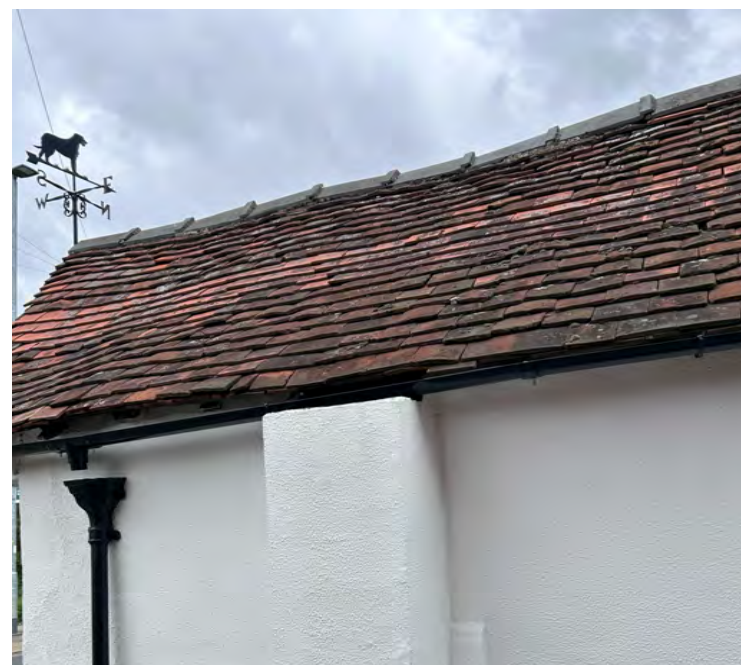
Fig 3.5 18th Century pitched roof with broken tiles
