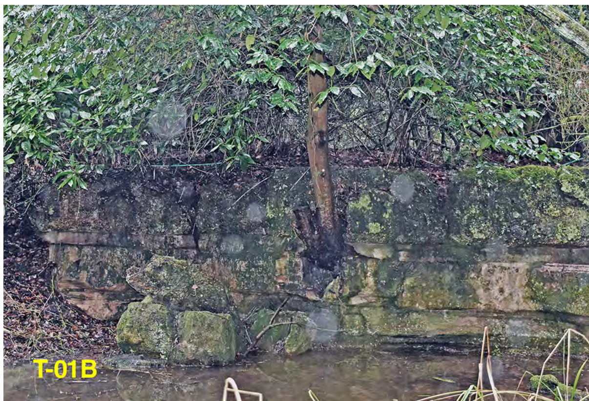
02: FRON VIEW OF SELF SOWN TREE (T-01 ) + DAMAGE TO FACE OF PULHAMITE
