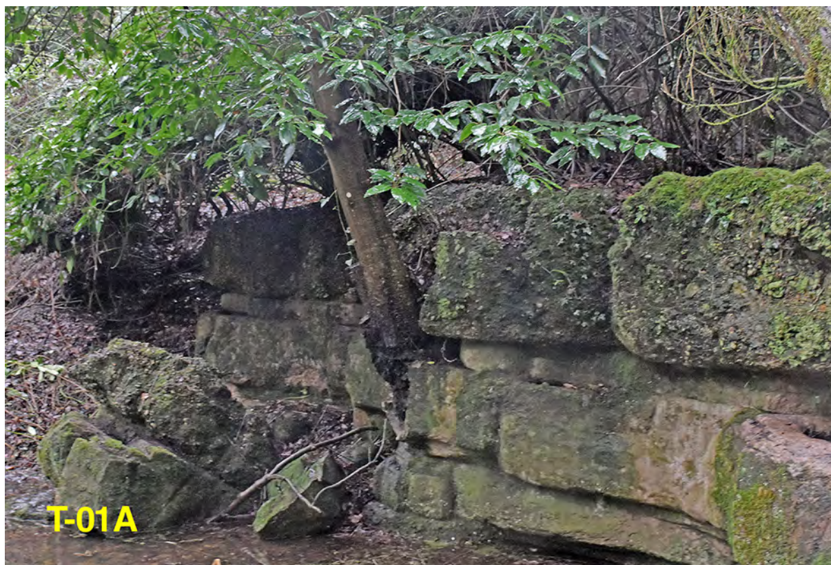
01: SIDE VIEW OF SELF SOWN TREE (T-01 )+ DAMAGE TO FACE OF PULHAMITE
