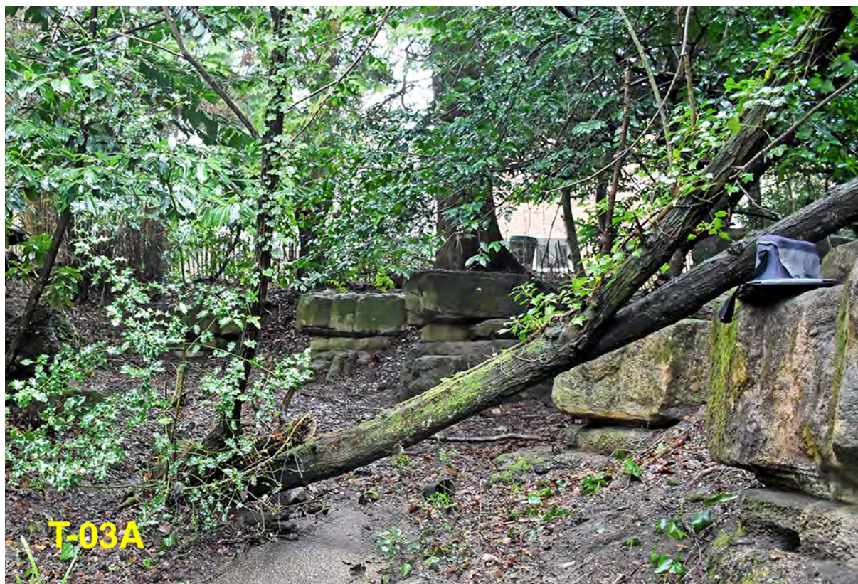
05: TREE T-03 FALLEN ACROSS PATH & NOW RESTING ON PULHAMITE
