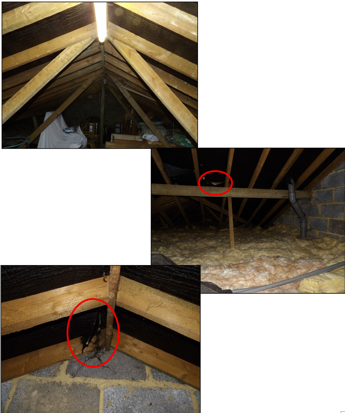
Figure 10. Example loft space and ripped bitumen felt. 372 Reading Road, Winnersh. 04.11.25
