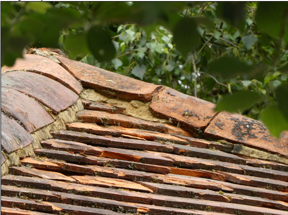
Figure 6. Example missing mortar from ridge tiles. Granary building at Stanlake Farm Cottage, Twyford. 03.06.25
