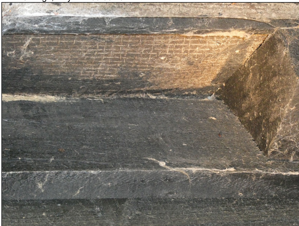
Figure 8. Example gaps between roof and wall plate. Granary building at Stanlake Farm Cottage, Twyford. 03.06.25
