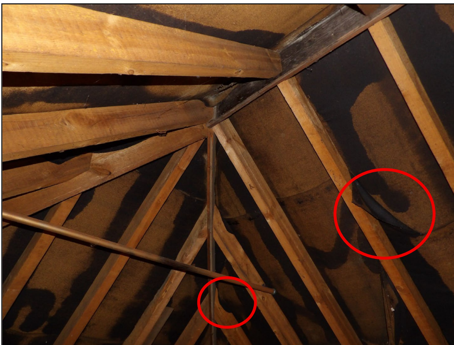
Figure 15. Hanging bitumen felt in loft. 6 Old Bath Road, Sonning. 20.05.25
