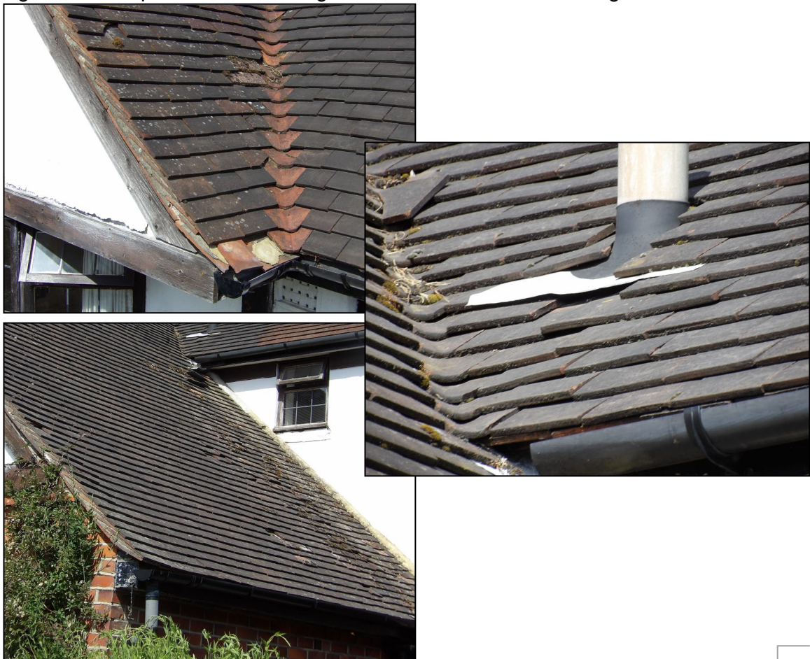
Figure 4. Example of raised/missing tiles. 6 Old Bath Road, Sonning. 20.05.25
