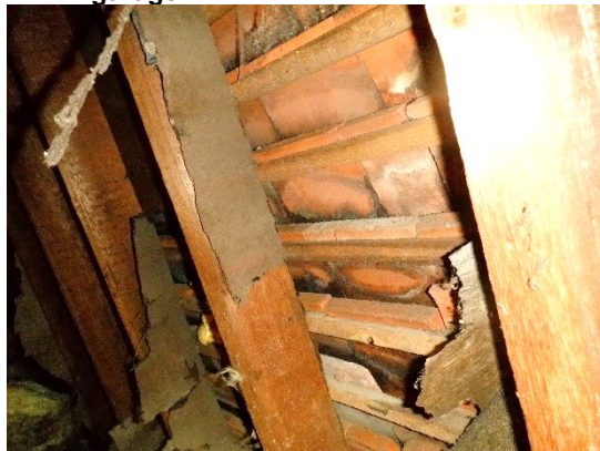
16. Internal view of the roof space lined with paper backed felt, which had numerous large tears.
