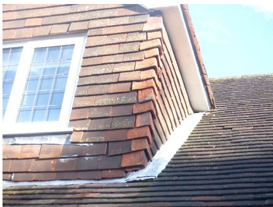
11. Numerous gaps behind the hanging tiles on the pitched roof dormer windows.
