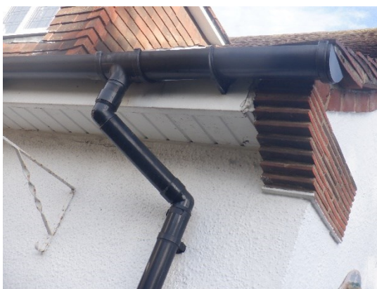
8. Upvc soffits tight at the eaves to the sides of the house.
