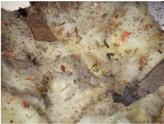
21. Pile of small bat droppings towards the front southern end of the roof.
