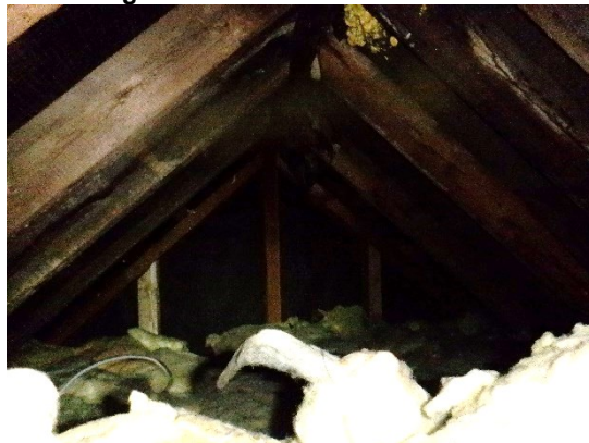
18. One of the dormer windows tightly lined with bitumen roofing felt.
