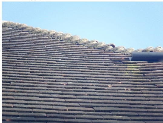
6. A few gaps under the hip tiles to the front of the house.
