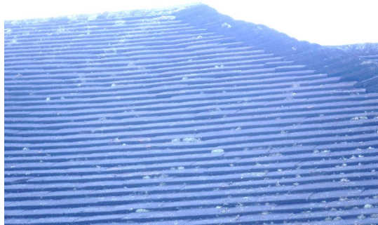
4. Gaps under some uneven roof tiles on the hipped roof to the front of the house.
