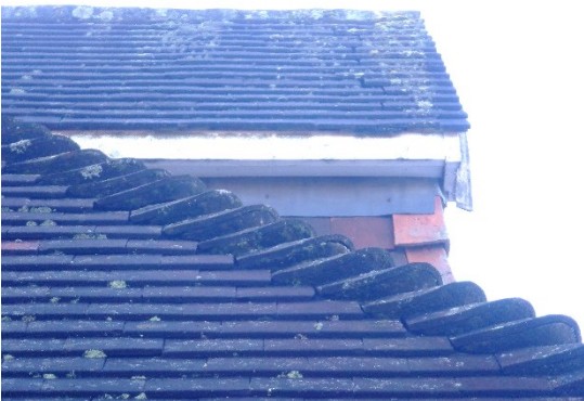
5. Lifted roof tiles on the dormer window to the eastern side of the house.
