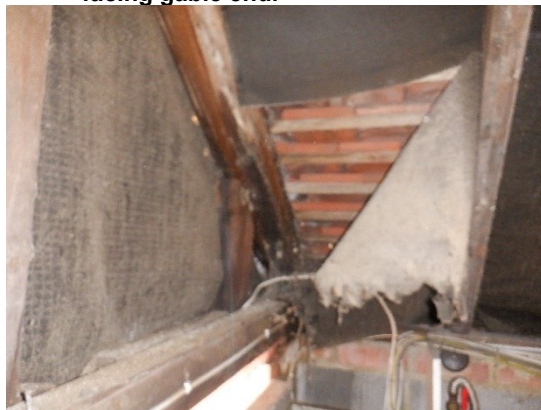
24. Roof of the garage with loose felt in places.
