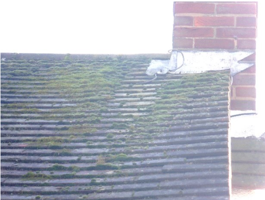
3. Lifted tiles on the verge at the rear of the house.
