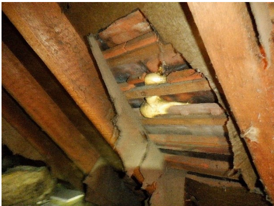
17. Large tear in roofing felt exposing the undersides of the roof tile.
