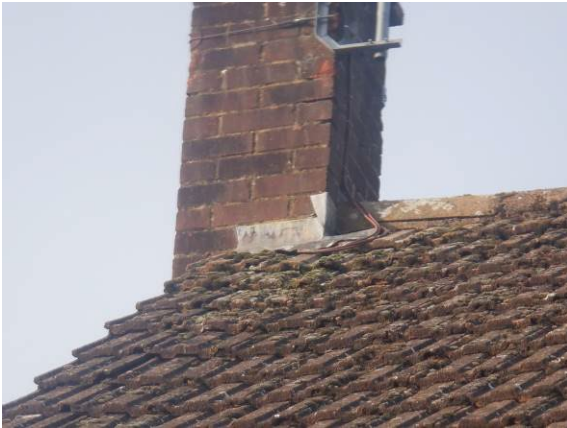
Photograph 7. Slight gap under lead flashing at western chimney (rear elevation).
