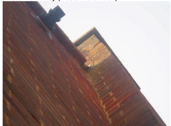
Photograph 10. Gap under lead flashing by eastern chimney (eastern elevation).
