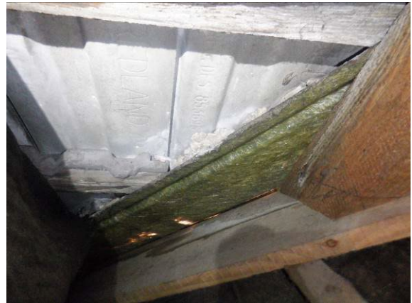
Photograph 16. Unlined roof at junction with front gable extension (roof void).
