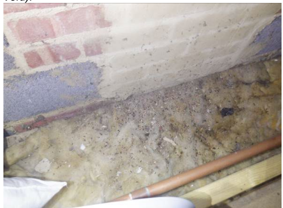
Photograph 22. Accumulation of small bat droppings at base of western gable (roof void).
