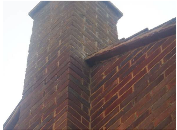
Photograph 8. Slight gap under lead flashing by western chimney (western elevation).
