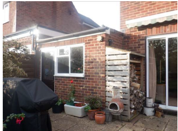
Photograph 12. Tight fascias on rear of garage (rear elevation).
