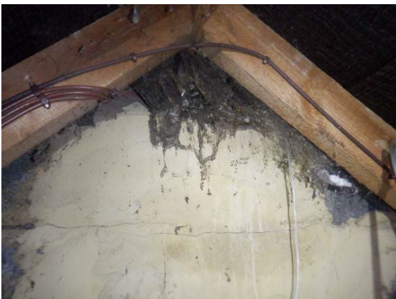
Photograph 21. Small bat droppings stuck to western gable (roof void).
