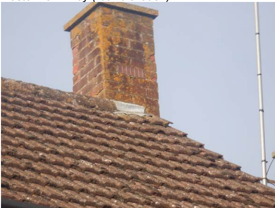
Photograph 9. Slight gap under lead flashing at eastern chimney (rear elevation).
