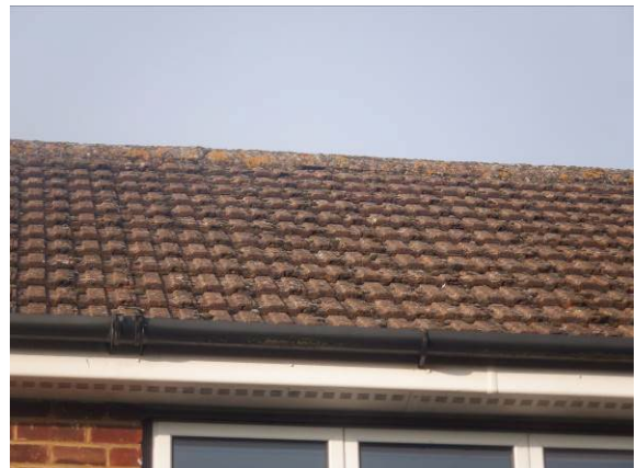
Photograph 4. Recess in ridge mortar (rear elevation).
