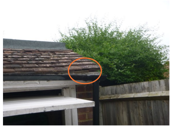
Photograph 14. Lifted tiles at one end of garage roof tiles (TN11).
