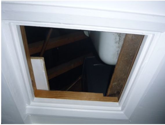
Photograph 25. Access limited by water tanks.
