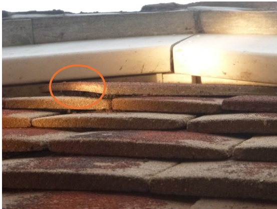
Photograph 7. Lifted hanging tiles on gable ends lifted in places (TN5-6).
