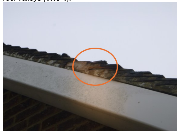
Photograph 6. Gaps in verge mortar ( TN2 ).
