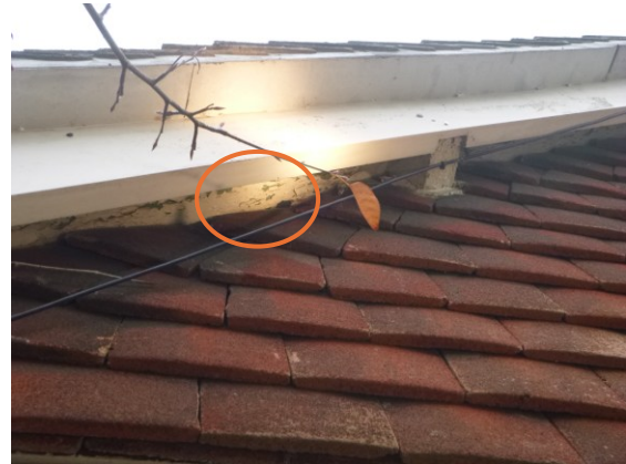
Photograph 8. Gaps at edges of gable end hanging tiles (TN5-6).
