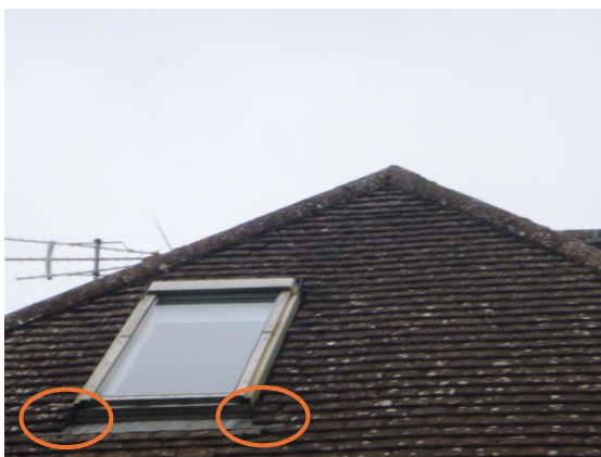
Photograph 11. Gaps around skylight (TN9).
