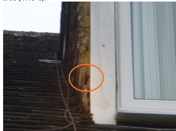
Photograph 10 Gaps in dormer mortar (TN8).
