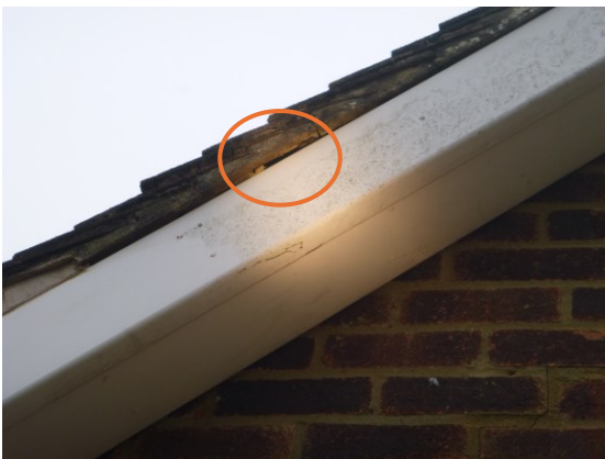
Photograph 5. Gaps between the verge mortar and uPVC bargeboard ( TN1 ).
