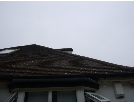
Photograph 3. Roof tiles mostly flat.
