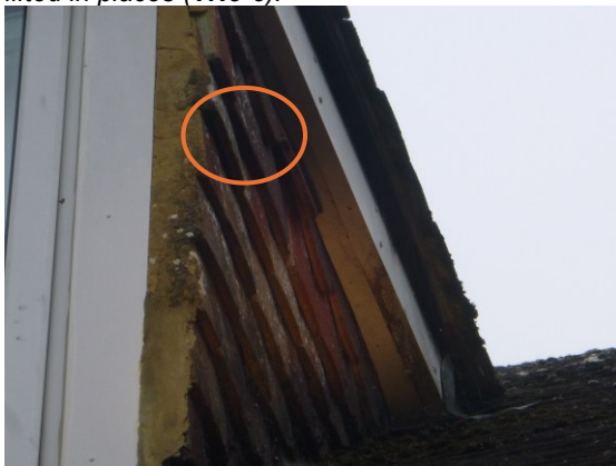
Photograph 9. Lifted hanging tiles on dormers (TN7).
