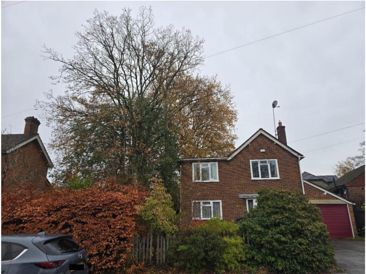
Photo 4 – Tree canopies in direct contact with roof of 81 Pinewood Avenue
