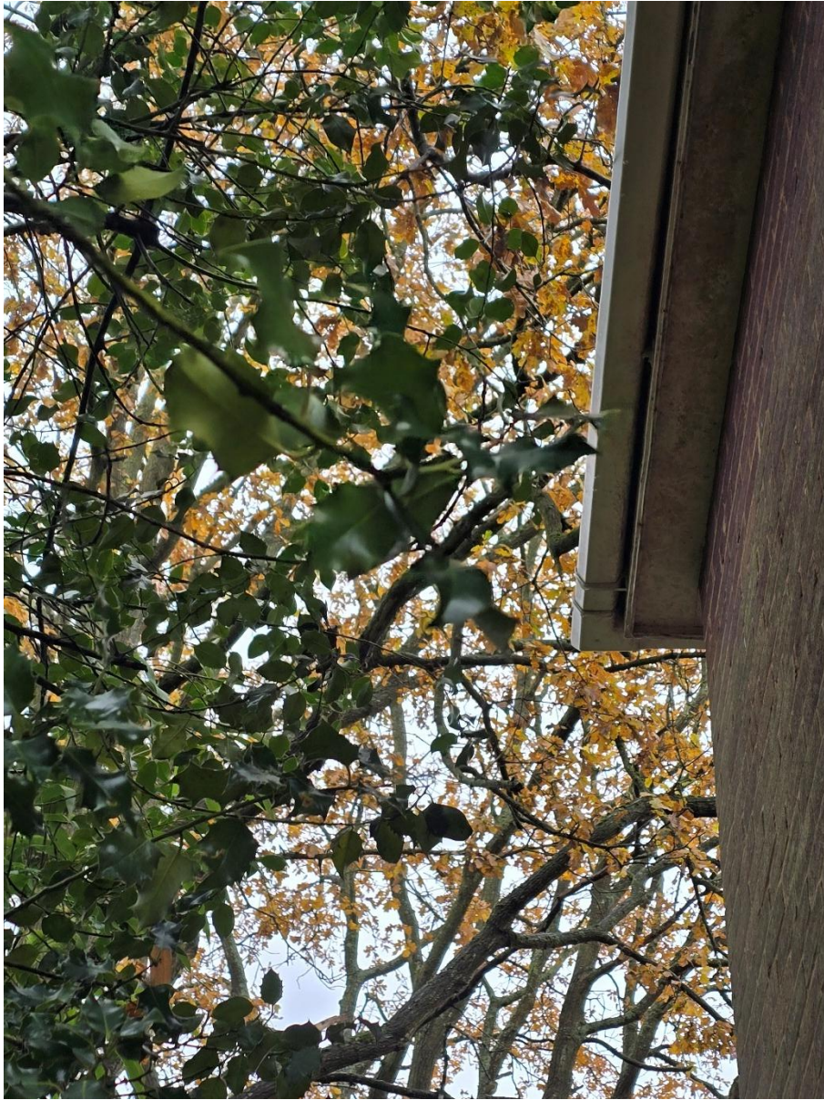
Photo 3 – Tree canopies in direct contact with roof of 81 Pinewood Avenue
