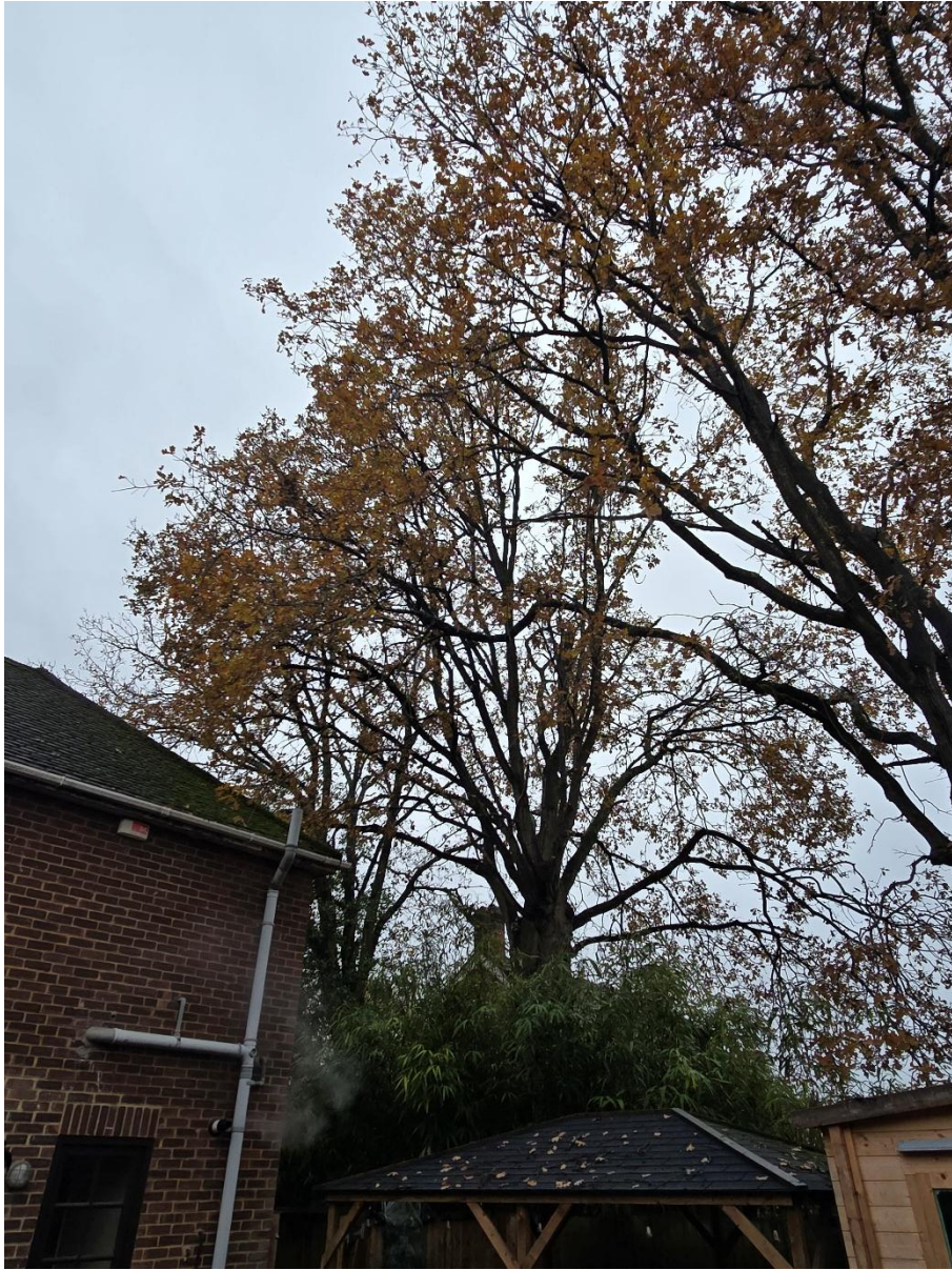
Photo 1 – Tree canopies in direct contact with roof of 81 Pinewood Avenue
