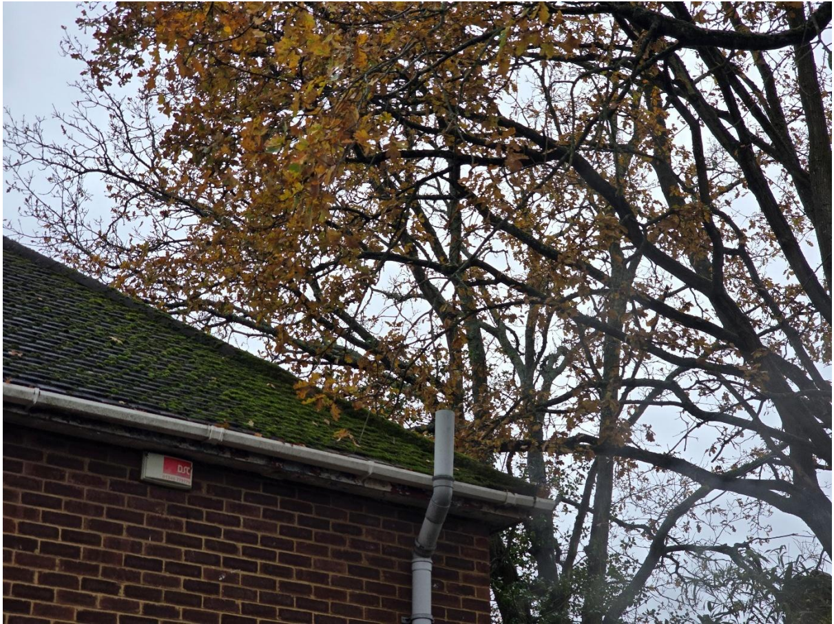
Photo 2 – Tree canopies in direct contact with roof of 81 Pinewood Avenue
