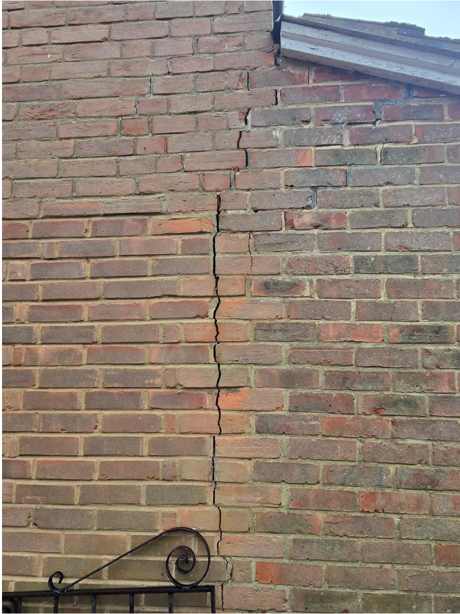
Photo 8 – Structural cracks on building of 81 Pinewood Avenue
