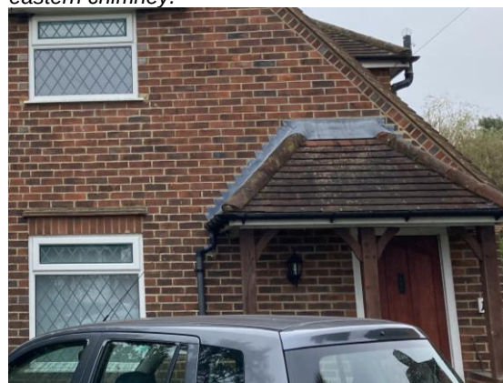
Photograph 8. Tight lead flashing throughout.
