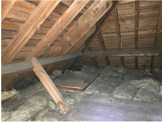
Photograph 11. Loose boards in places over fibreglass insulation.
