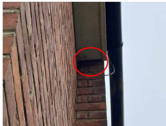
Photograph 6. Small gap behind soffit around eastern chimney.
