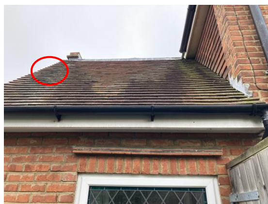
Photograph 4. Slightly lifted tile on sloping roof near the front entrance.
