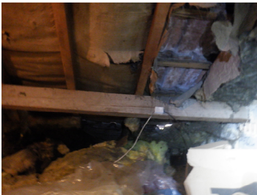
Photograph 9. Bituminous paper and horse hair lining with tears throughout the void (roof void).
