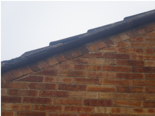
Photograph 5. Gap in verge mortar (western elevation).
