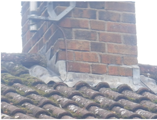
Photograph 5. Small gap in ridge mortar and lifted lead flashing on western side of chimney (front elevation).
