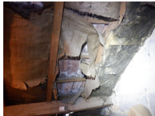
Photograph 10. Section of roof on western side of roof void that was lined with fibreglass along the verge (roof void).
