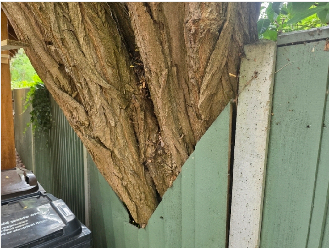
T01 - Visible damage to fence and post
