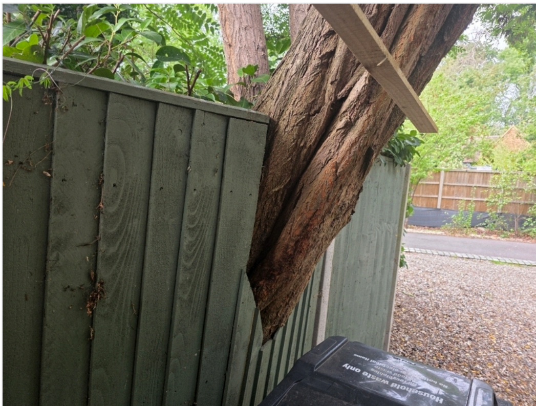
T01 - Moving stem visibly pushing fence out of line
