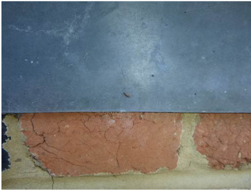
Photograph 11. Small bat dropping stuck to lead flashing (rear elevation).
