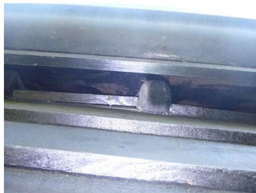
Photograph 10. Potential bat ingress behind lifted weatherboard (western elevation).
