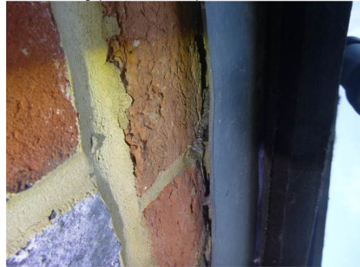
Photograph 14. Potential bat ingress behind lead flashing (rear elevation).
