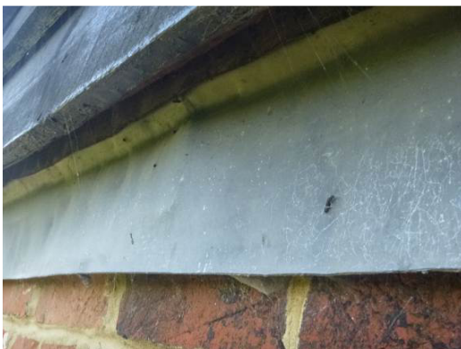
Photograph 9. Small bat droppings stuck to lead flashing (western elevation).
