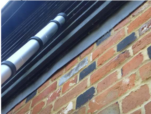
Photograph 13. Potential bat ingress behind lead flashing (rear elevation).
