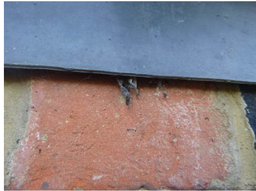
Photograph 12. Small bat droppings caught behind lead flashing (rear elevation).
