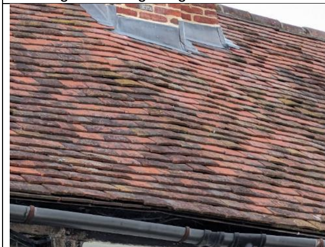
Photograph 4: Gaps under cambered tiles
