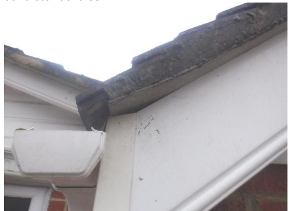
Photograph 11. Superficial gap between uPVC fascia and verge mortar (front elevation).
