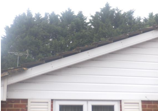
Photograph 8. Missing verge mortar across the front gable (front elevation).
