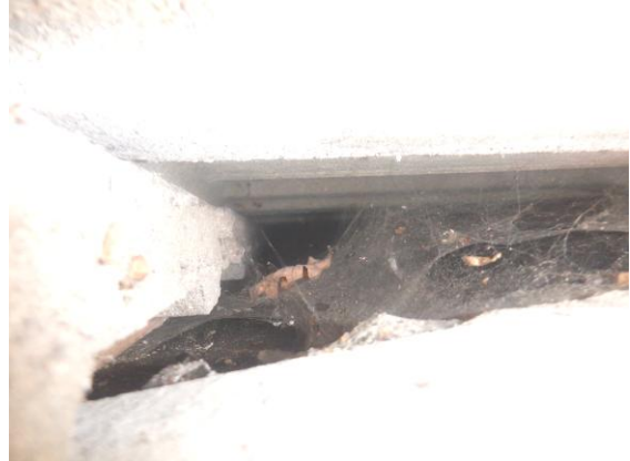
Photograph 9. Open gap between roof lining and concrete roof tiles.
