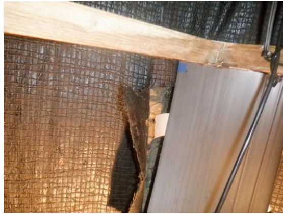
Photograph 18. Large tear in bitumen felt with roof tiles visible.
