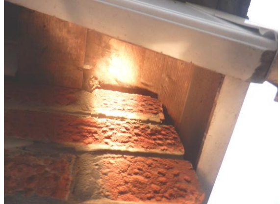
Photograph 15. Heavily cobwebbed gap behind uPVC fascia (front elevation).
