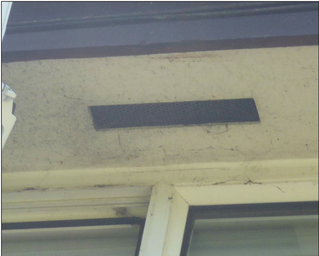
Figure 8. Ventilation holes in soffit boxes. 21 Hubbard Close, Twyford, 30.07.24
