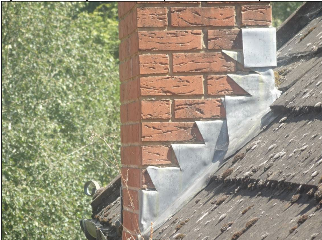
Figure 6. Lead flashing around the chimney. 21 Hubbard Close, Twyford, 30.07.24
