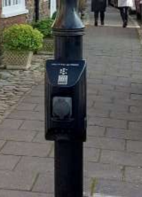
FIGURE 215 STANDARD LIGHTING COLUMN WITH EV CHARGING POINT
