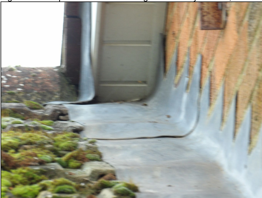
Figure 7. Example sealed lead flashing. 9 Northbury Avenue, Ruscombe. 21.01.25
