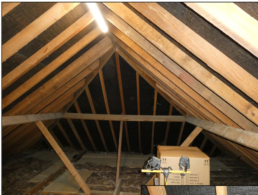
Figure 11. Example of loft space and bitumen lining to tiles. 10 South Close, Wokingham. 15.04.25
