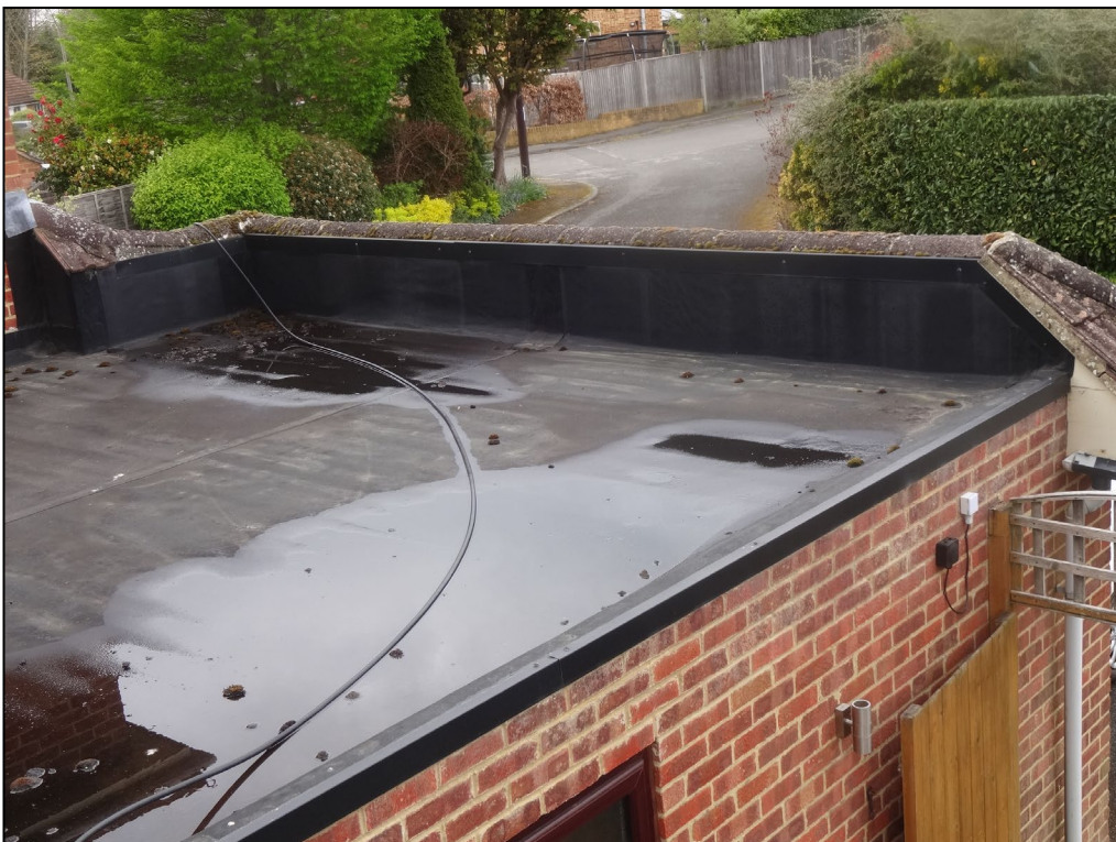
Figure 8. Flat roof membrane covered section of garage. 10 South Close, Wokingham. 15.04.25
