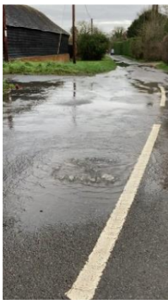
Thames Water pumping station ineffective
