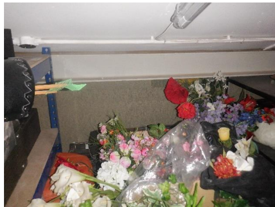
Photograph 20. Roof void 1 boarded up to the eaves.
