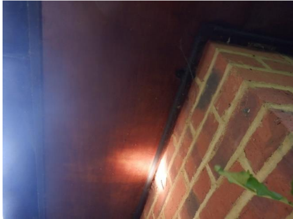
Photograph 17. Small gap behind overhanging eaves (northern elevation).
