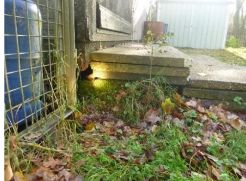
Photograph 8. Gaps around the patio slabs on the steps of the scout hut.
