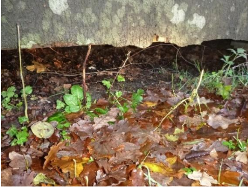
Photograph 7. Gap under the northern side of the scout hut.
