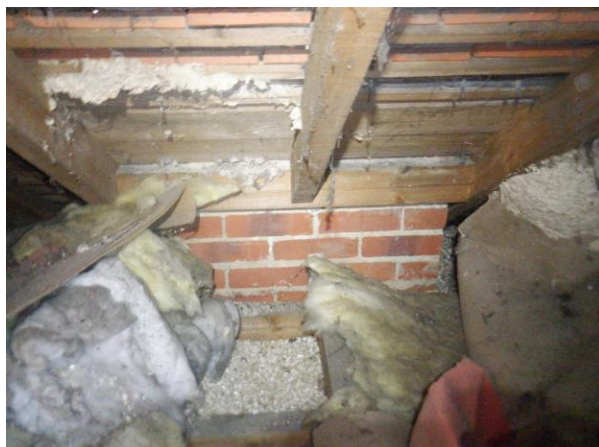
Photograph 15. Wasp nest at the base of the brickwork chimney.
