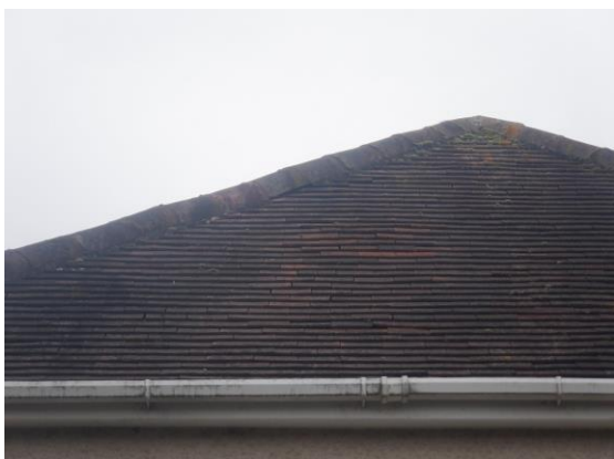
Photograph 3. Raised roof tiles and crumbling hip mortar (rear elevation).
