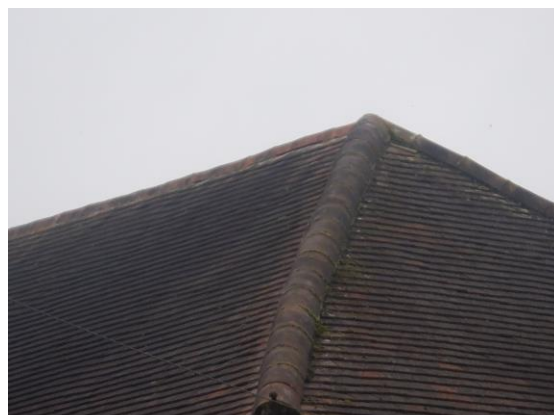
Photograph 4. Crumbling ridge mortar (south elevation).
