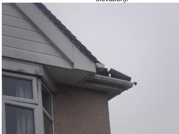
Photograph 5. Hip tile coming away from roof (front elevation).
