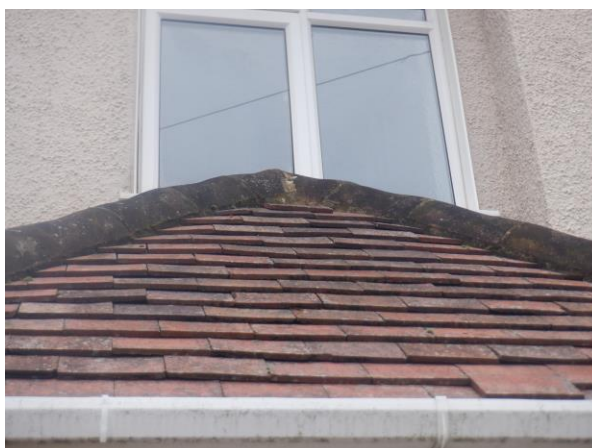
Photograph 9. Clay tiles lifted on front porch (front elevation).
