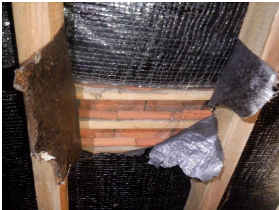
Photograph 11. Tear in bitumen felt at the western end of the void, with roof tiles visible (roof void).
