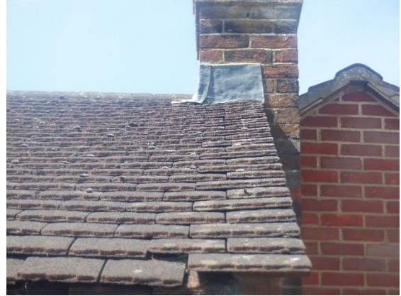
Photograph 2. Slightly separated verge tiles at the north western end of the roof; no bat evidence during endoscopic inspection.
