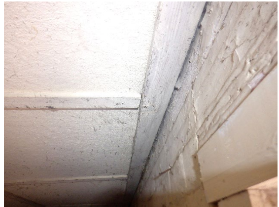
Photograph 12..Slight gap between board ceiling
