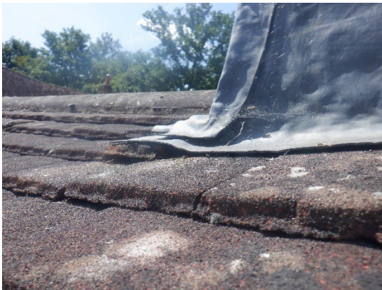
Photograph 3. Gap under lead flashing at base of chimney at the north western end; no evidence of bats during endoscopic inspection.
