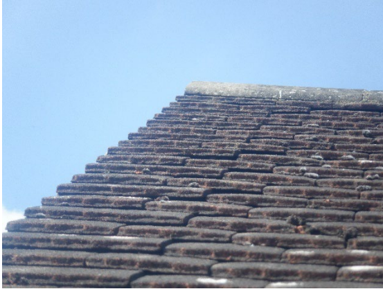
Photograph 5. Slightly separated verge tiles at the south eastern end of the roof; no evidence of bats during an endoscopic inspection.
