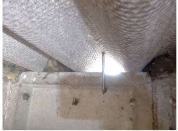
Photograph 14. Daylight between corrugated sheets and walls.
