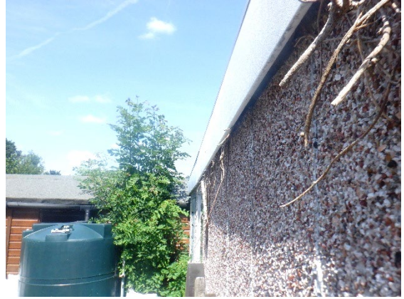
Photograph 10. Large gap behind fascia (southern side).
