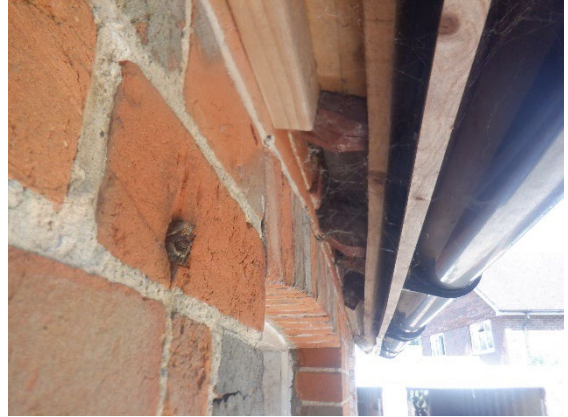
Photograph 6. Open eaves on north eastern side largely cobwebbed.
