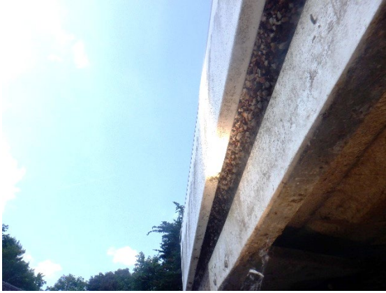
Photograph 9. Large gap behind fascia (eastern side)
