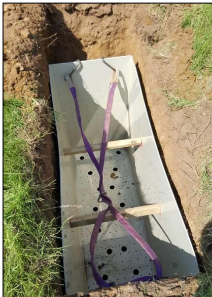
SA-03 with soakaway crate
