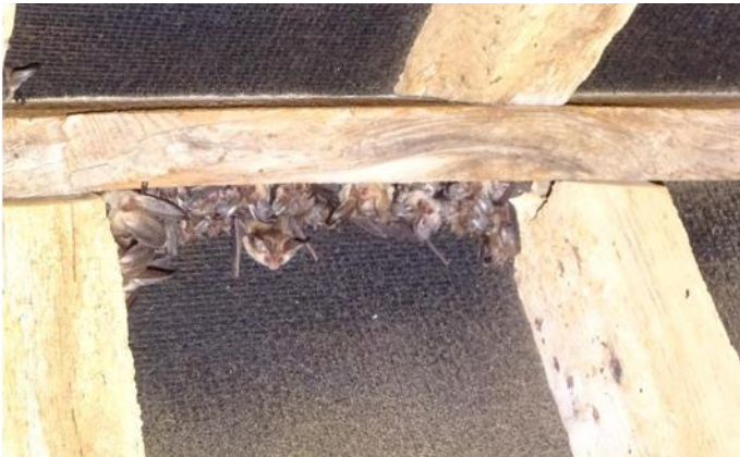
Figure 1: Maternity roost of brown long-eared bats within the loft space of B1 during the PRA (Arbtech, 2022). Furthermore, approximately 200 droppings were observed on the floor of the loft, directly below the ridge line.
