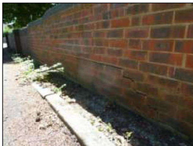
Photograph 1: Cracking at base of wall, South Lodge. 30.6.2015.
