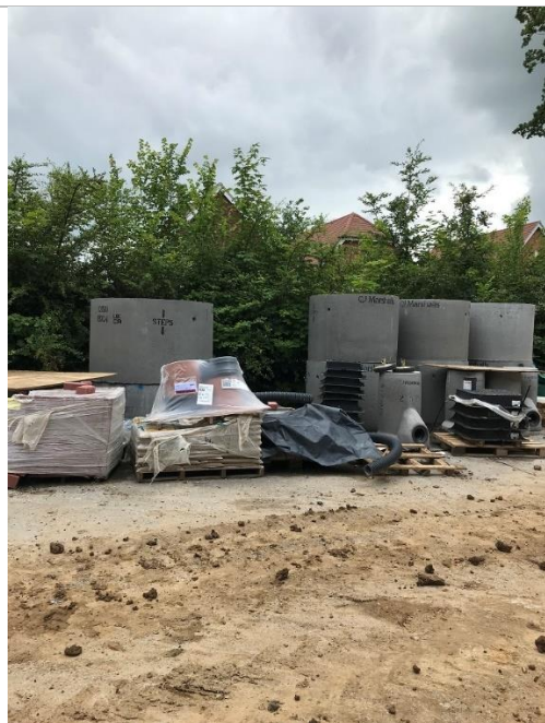
Photo 5. Car park used as storage area
