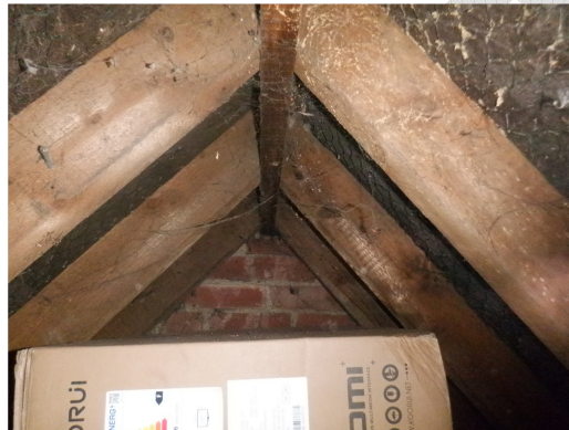
Photograph 28. Gap between timbers and brickwork gable (Roof void 3).
