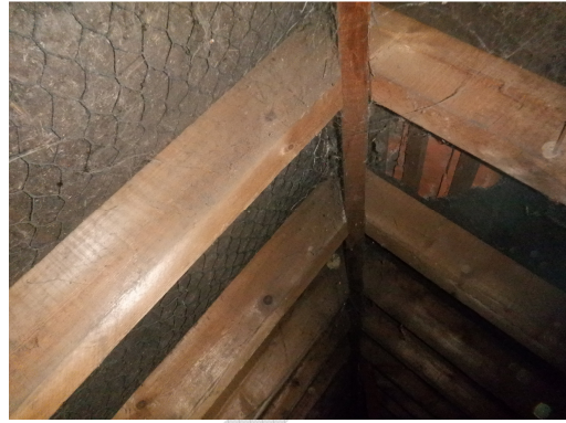
Photograph 27. Torn horsehair felt covered by a wire mesh with roof tiles visible (Roof void 3).
