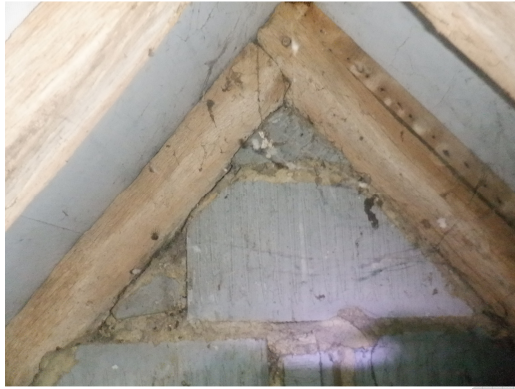
Photograph 24. Timbers sealed to the western blockwork gable (Roof void 2).
