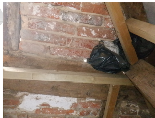
Photograph 23. Gaps within the single-skin eastern brick gable with daylight visible (Roof void 2).
