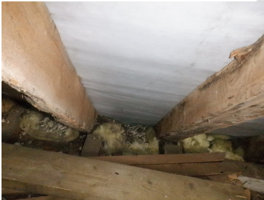
Photograph 24. Brickwork and daylight visible with the eastern eaves (Roof void 2).
