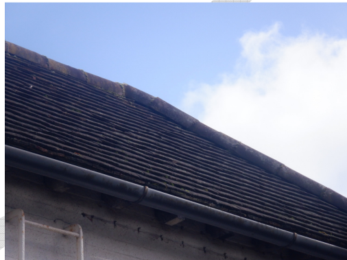
Photograph 9. Crumbling hip mortar (west elevation of rear extension).
