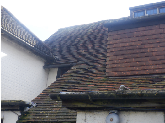
Photograph 3. Frequently lifted/uneven clay roof tiles (rear elevation).
