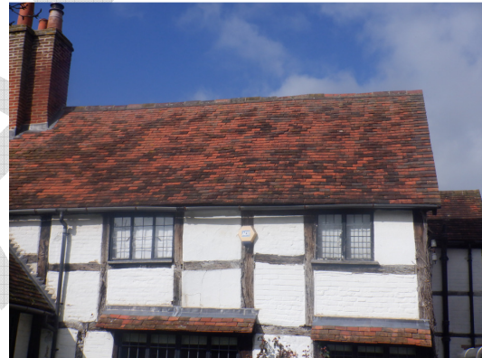
Photograph 4. Frequently lifted/uneven clay roof tiles (front elevation).
