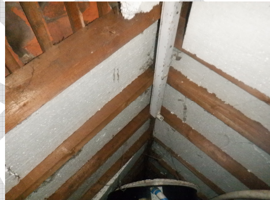
Photograph 17. Roof tiles visible behind sections of missing polystyrene (Roof void 1).
