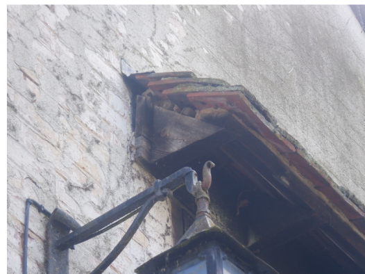
Photograph 6. Gap between clay roof tiles & timber battens (rear elevation).
