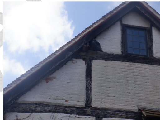
Photograph 14. Gaps behind the timber fascia and at the edges of the window & timbers within the painted brickwork gable (east elevation).
