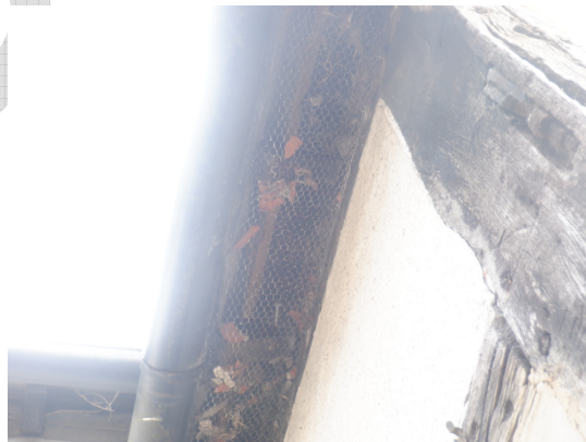
Photograph 15. Chicken wire situated at the eaves of in places (west elevation).
