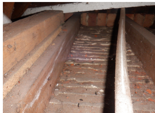
Photograph 19. Rat droppings throughout the void (Roof void 1).
