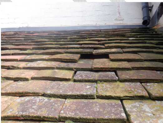
Photograph 5. Lifted and missing clay roof tiles on the catslide roof (west elevation)
