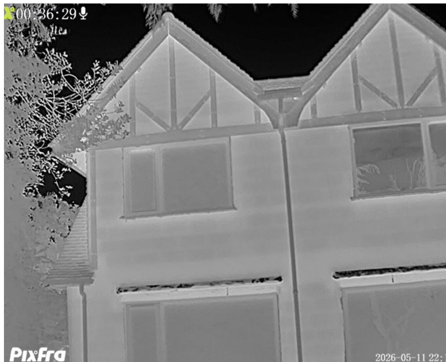
Pixfra ARC A613 at Surveyor Location 1.
