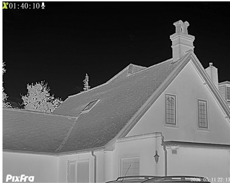
Pixfra ARC A613 at Surveyor Location 3.
