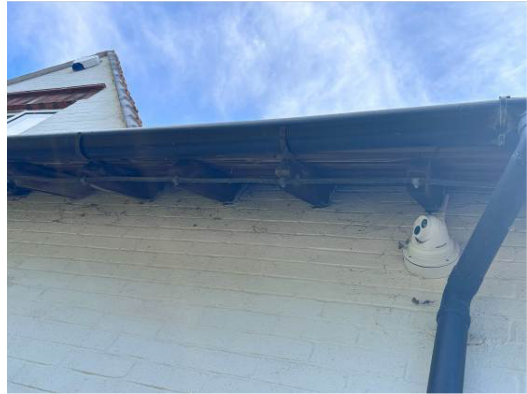
Photograph 7. Timbers tight along the eaves to the front of the property
