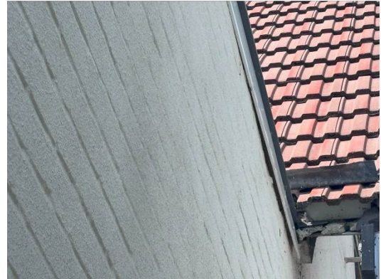
Photograph 12. Gap of limited extent along the eastern side of the rear extension.
