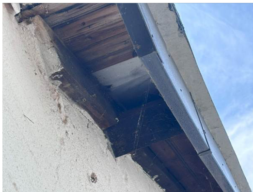
Photograph 8. Gaps at the base of the eaves at the eastern side of the property.
