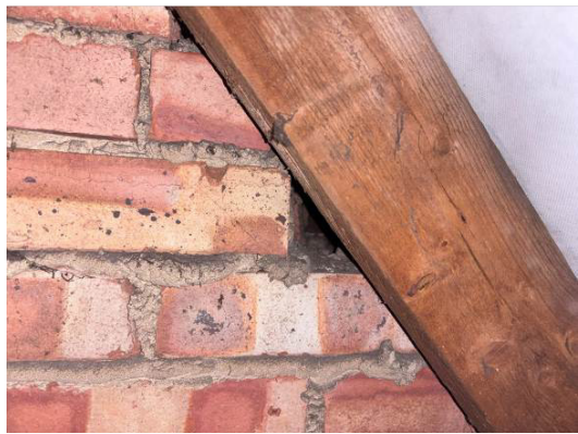
Photograph 18. Gaps around the brickwork at the eastern gable end.
