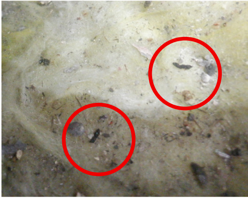
Photograph 20. Small bat droppings found on top of the fibreglass in the void. r
