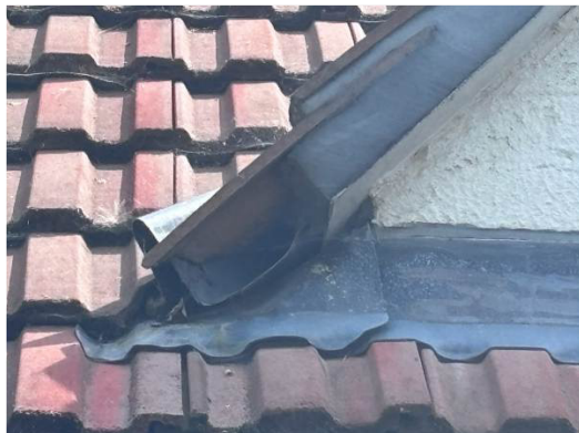
Photograph 10. Gap in lead flashing to the front of the house.
