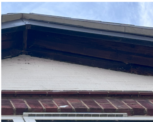
Photograph 9. Gaps between the timbers at the eastern side of the property.
