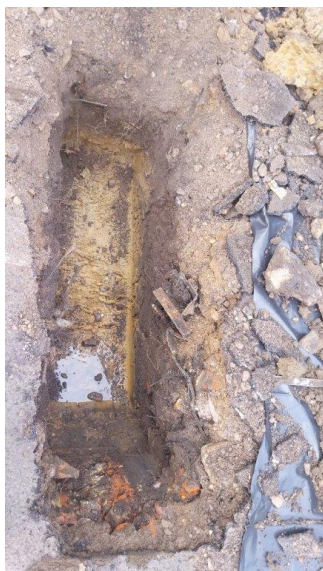
Photograph 5 - Looking down at water seepage encountered at 0.8m bgl within TP01.
