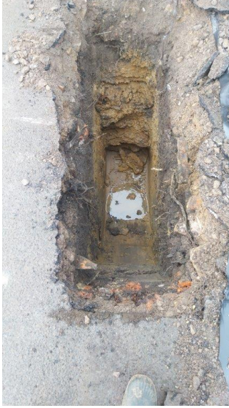
Photograph 7 - Looking down at water seepage encountered at 1.4m bgl within TP01.
