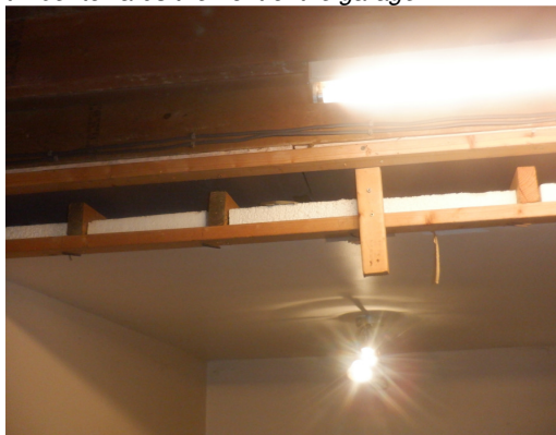
Photograph 22. Polystyrene in section towards the rear of the garage.
