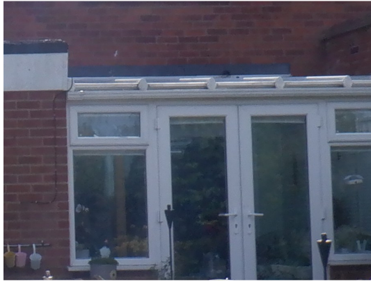
Photograph 12. Tight uPVC and glass conservatory
