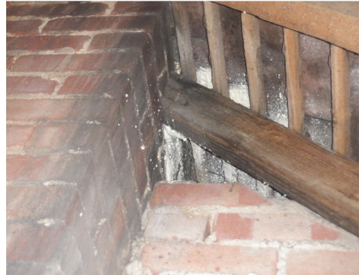
Photograph 16. Small gaps with visible daylight at the apex of the chimney.
