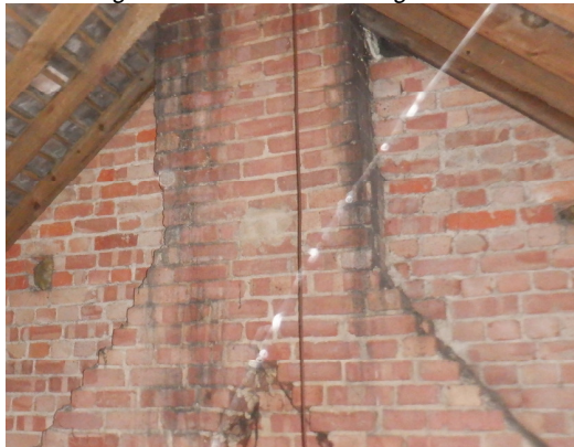
Photograph 17. Expanding foam within the brick work visible either side of chimney.
