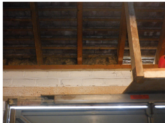
Photograph 19. Unlined roof to the front of the garage with fibreglass at the eaves.
