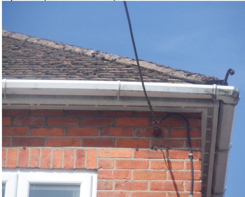
Photograph 5. Small gap beneath hip tile at the base of the roof (front elevation)
