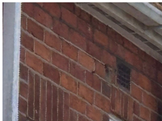
Photograph 7. Small hole in northern side of the house which was an active house sparrow nest.
