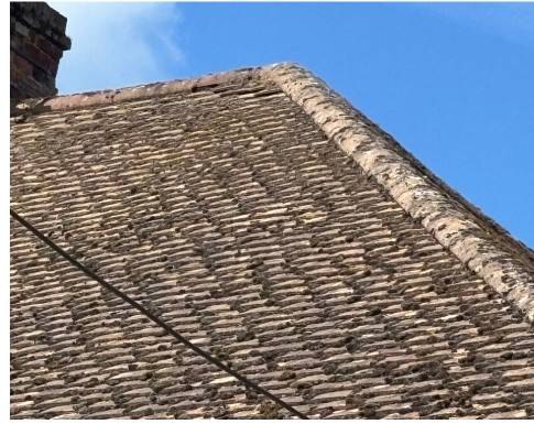
Photograph 4. Small gaps beneath the roof, ridge and hip tiles (front elevation)
