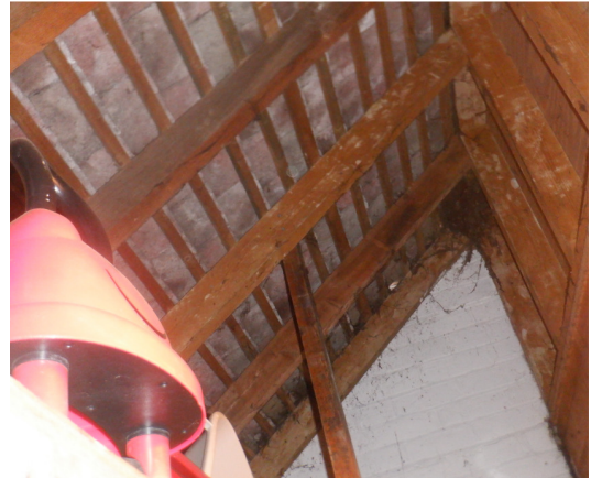
Photograph 21. Roof heavily cobwebbed in the garage.
