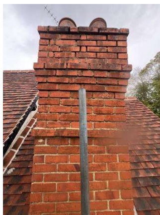
Photograph 03 – Pronounced lean from front to back
