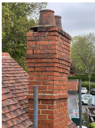
Photograph 02 – Poor / missing pointing and loose brickwork to the head of the chimney
