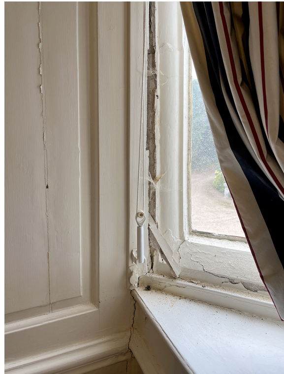
1st floor north bay Bay detaching from front wall
