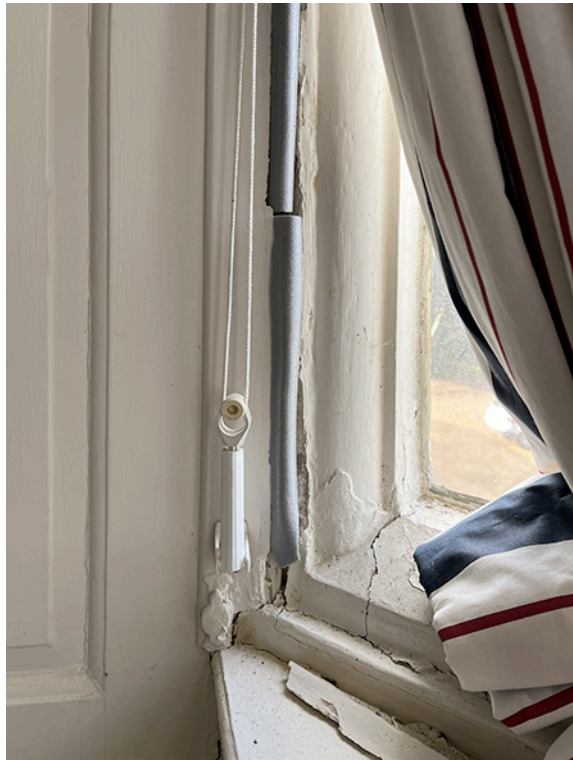
1st floor north bay Close up showing foam pipe insulation stuffed into gap between window and wall
