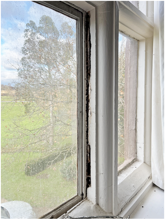
1st floor north bay Mullion and casement windows Casements do not close and frame is no longer weatherproof
