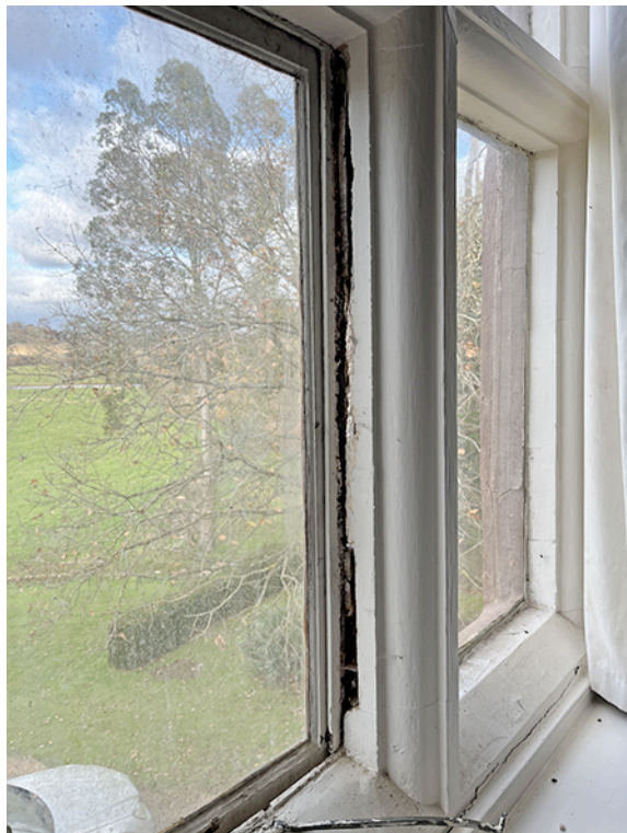
1st floor north bay South east mullion showing poor quality cement based stonework repair
