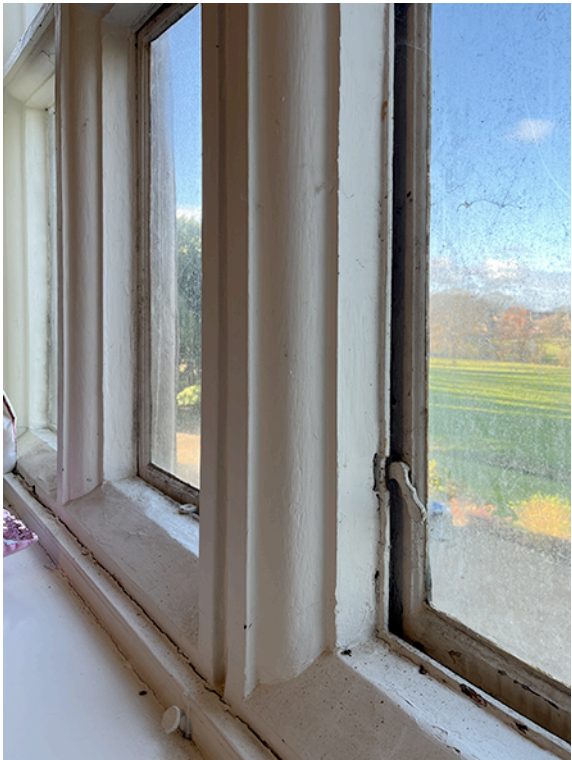
1st floor north bay Central mullion and casement windows Casements do not close and frame is no longer weatherproof
