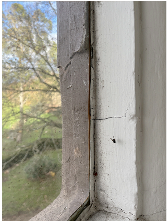
1st floor north bay Close up showing fixed light fixing and poor cement based repair to external stonework which intself has now failed
