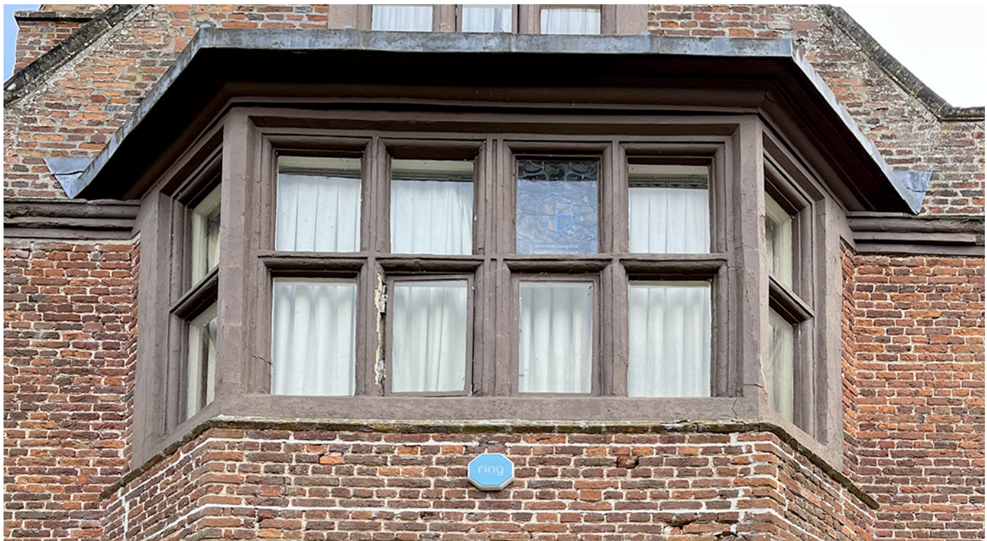
1st floor north bay stonework in very poor conditon, with extensive cement based repairs (now in very poor condition) and inappropriate paint finish
