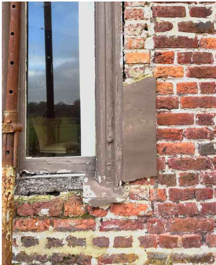
Left hand bay ground floor detail showing timber window and surround, timber cill, and render side panel, all in very poor condition. Also note tuck pointing now disappeared, with cement mortar repairs
