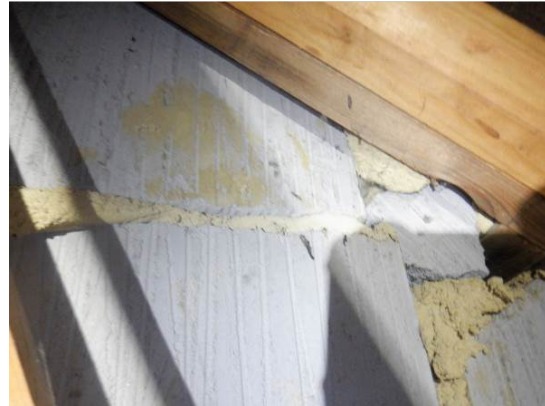
Photograph 19. Gaps between the block work at bitumen roofing felt.
