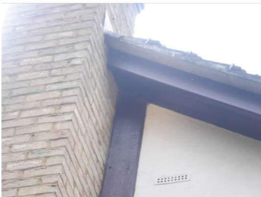
Photograph 5. Gap between timber and chimney breast (western elevation).
