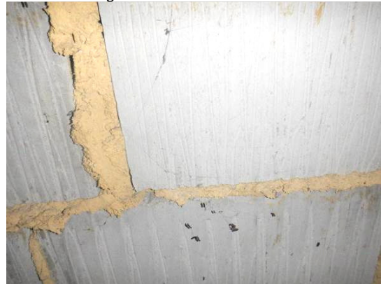
Photograph 21. Small bat droppings stuck on the east facing gable end wall.
