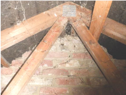
Photograph 25. Heavily cobwebbed external gable end wall (eastern elevation)
