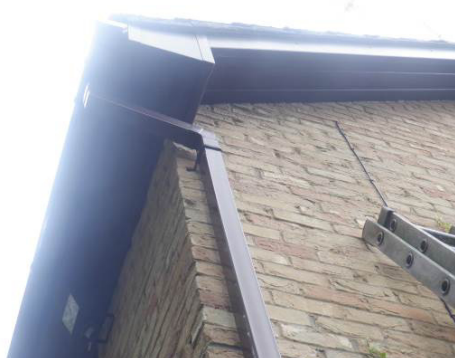
Photograph 7. Sealant present under the soffits (western elevation).
