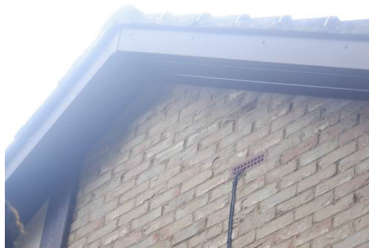
Photograph 8. Gap between the soffit and wall (eastern elevation).
