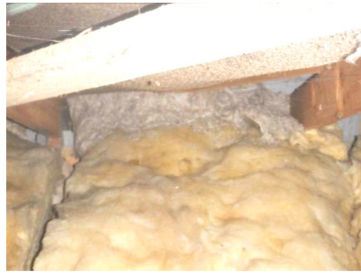
Photograph 17. Blockwork at eaves and wasps nest present (roof void).
