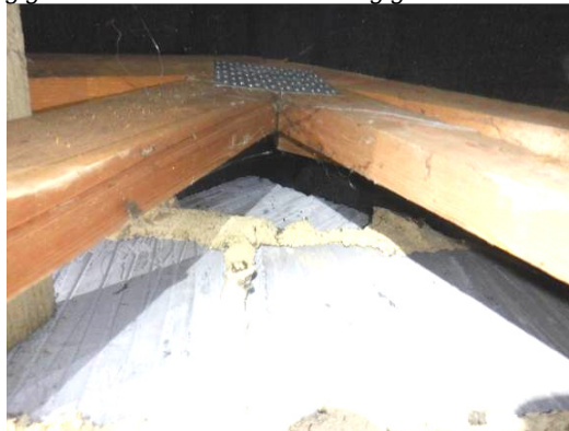
Photograph 22. Small bat droppings stuck on the west facing gable end wall.
