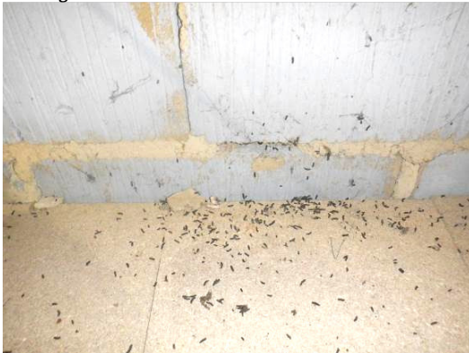
Photograph 20. Accumulation of small sized bat droppings at the east facing gable end.
