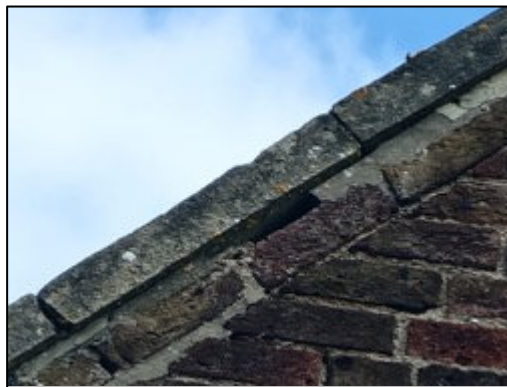
Figure 28 – Gaps under stone coping where mortar is missing.
