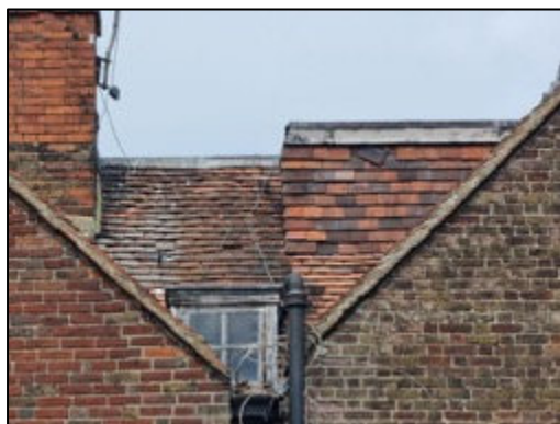
Figure 24 – lifted roof tiles on the southern roof face and slipped hanging tiles.
