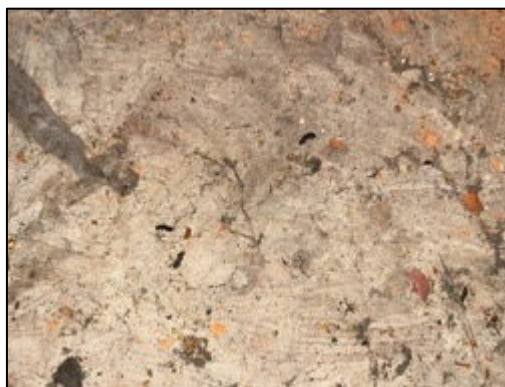
Figure 35 – Scattered long-eared bat droppings in the roof void.
