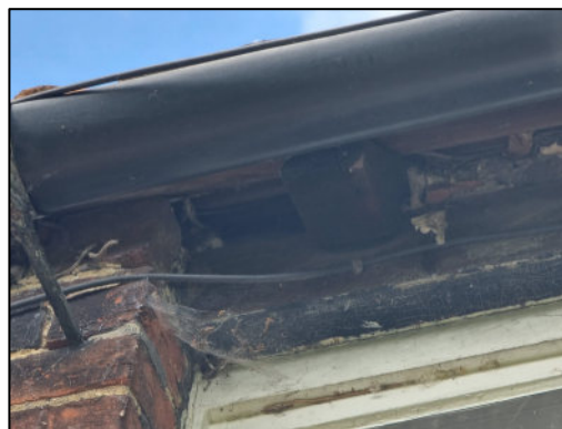
Figure 34 – Gap in the eaves above the northern elevation.
