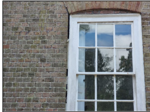
Figure 27 – Crevices around the window frames where mortar has fallen away.
