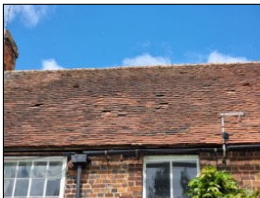
Figure 33 – Southern roof face of Rose Cottage with slipped roof tiles.
