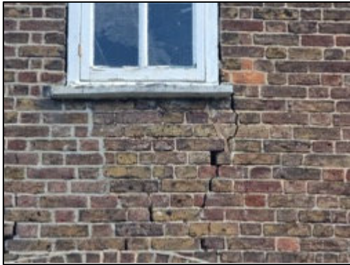
Figure 26 – Cracks in the western elevation of the house.
