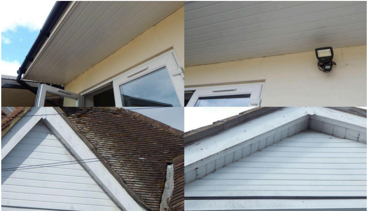
Image 7 – View of eaves coverings to demonstrate condition
