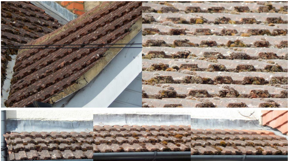
Image 6 – Example images across the main tiled roof coverings to demonstrate condition
