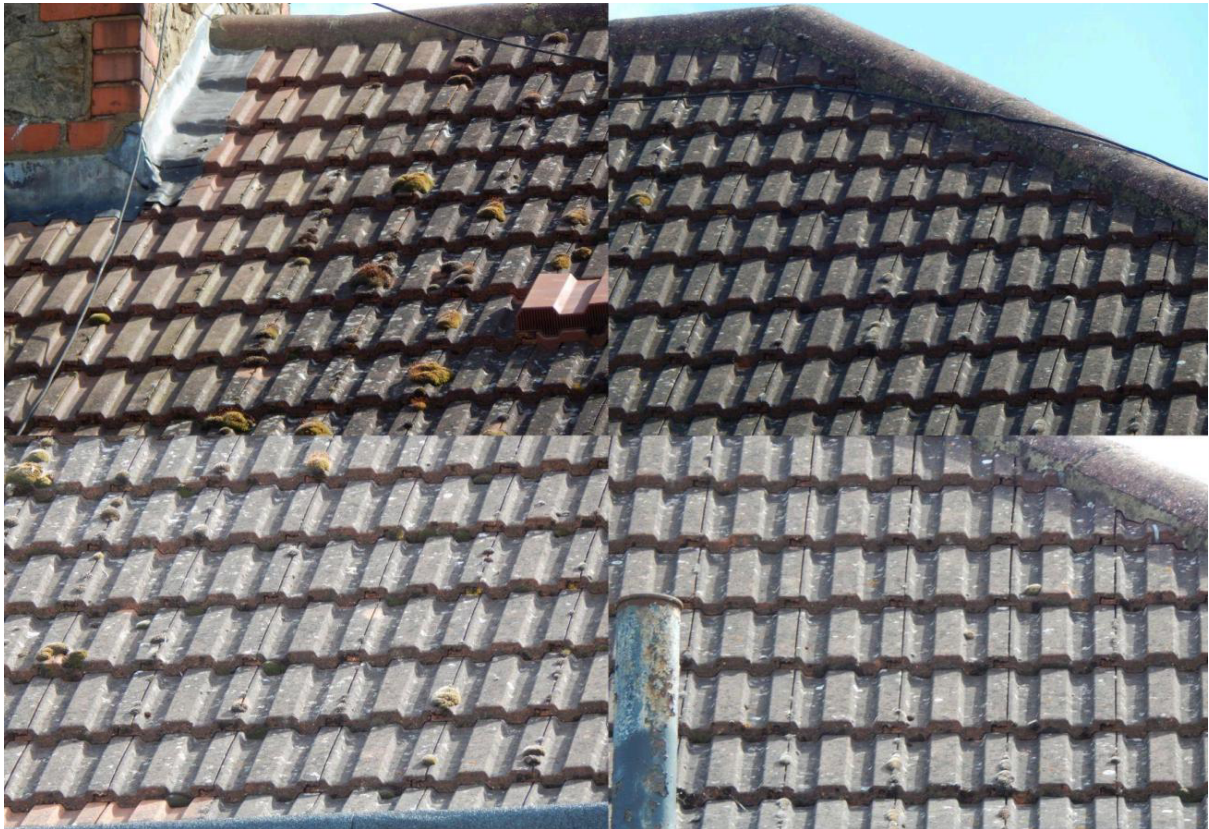
Image 5 – Example images across the main tiled roof coverings to demonstrate condition
