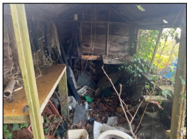
Image 6: One of the dilapidated sheds on site.
