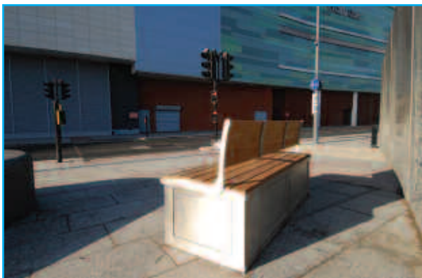
Bench containing traffic signal controller
